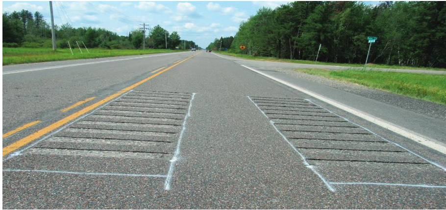
Figure 93. Photo. Wheel path transverse rumble strip.
