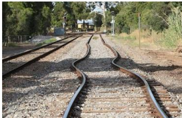
Figure 3 Buckling of tracks in lateral direction (Knapton 2015)
