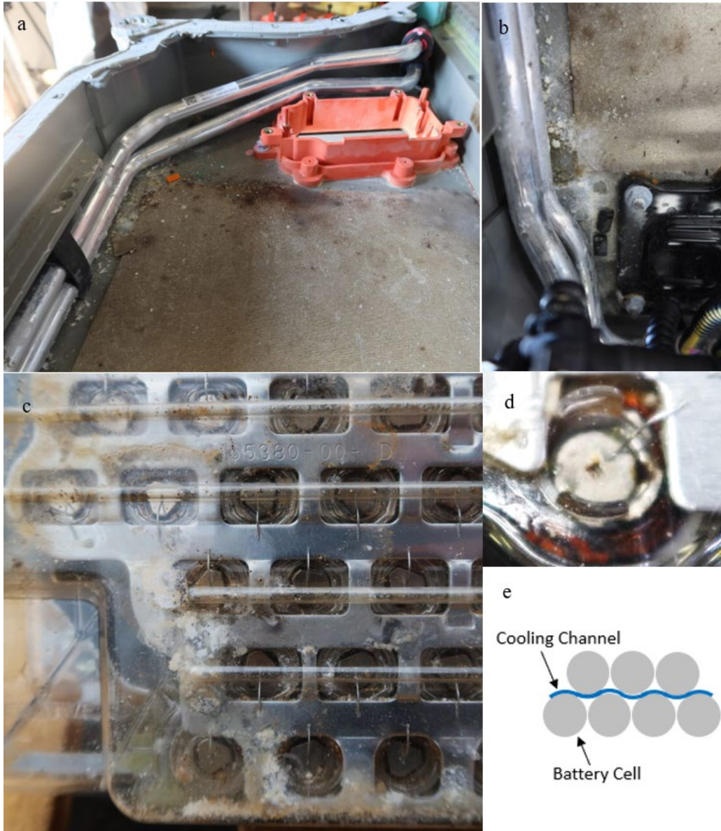
Figure 49. Image showing the impact of water damage that may have contributed to an isolation fault in Vehicle 9: (a) aluminum coolant tube at front of pack, (b) corrosion build up between aluminum coolant tubes and pack chassis, (c) corrosion on current collectors because of ingress, (d) corrosion on battery cell, and (e) cell-cooling arrangement
