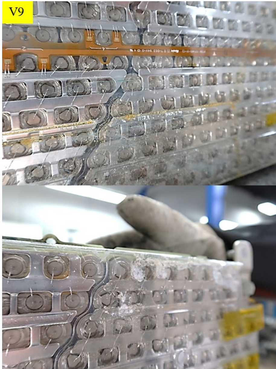
Figure 47. Vehicle V9, module M9 (i.e., the upper module in the penthouse), showing watermarks, contamination, and corrosion
