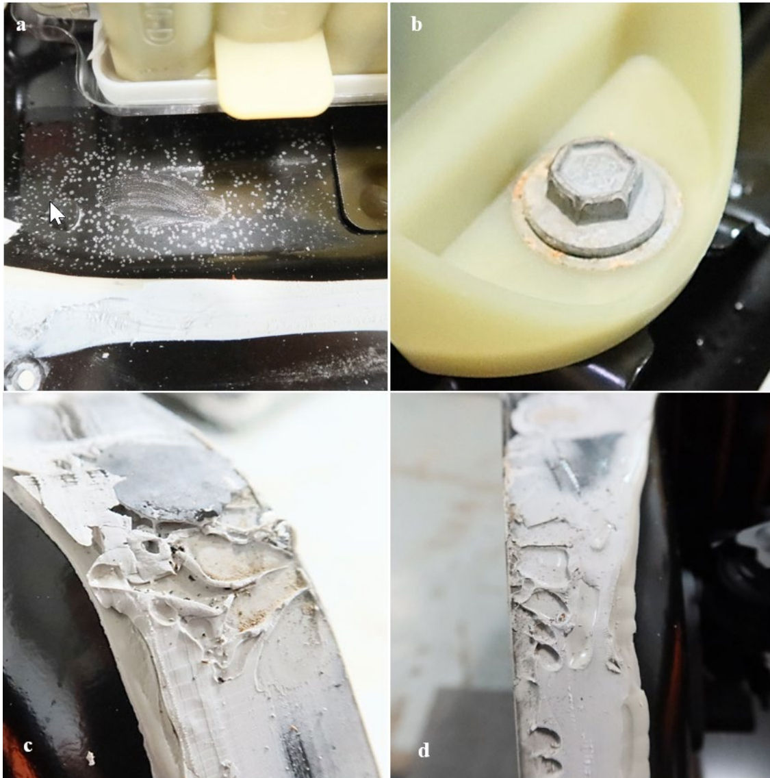
Figure 30. Observation inside the V10 battery pack: (a) water residue (note smear) underneath battery module, (b) corroded module fastener, (c) defective appearance of the lid seal, and (d) air pockets in another area of the seal, which did not result in ingress (bottom right)
