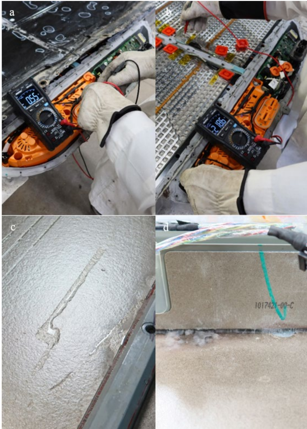
Figure 48. V9 battery pack: (a) measuring the external HV terminals with the contactor open; (b) measuring the voltage between battery module M1 and the battery chassis; (c) water on the floor of the module cavity; and (d) mold along the center spine of the tray
