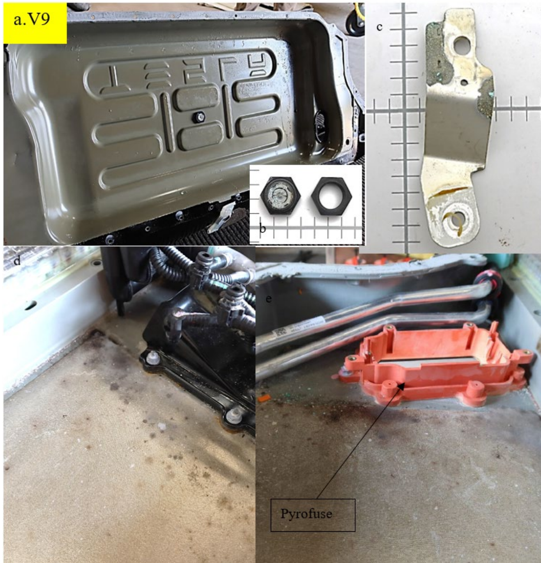
Figure 42. Vehicle V9 penthouse area: (a) interior face of penthouse lid, covered in condensation, (b) heavily corroded vent, (c) corrosion on the pyro-fuse bus bar, and (d, e) water marks, contaminants, and mold on battery penthouse floor
