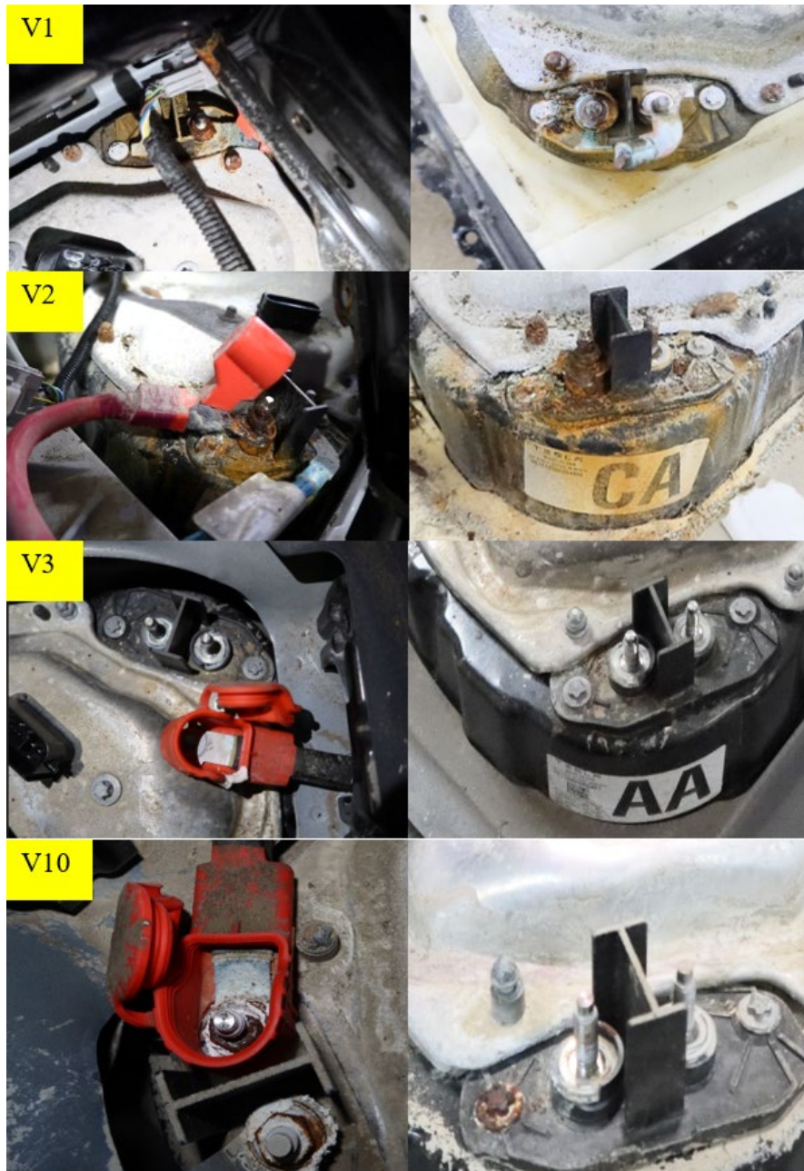
Figure 22. The front-right corner of the penthouse compartment shows two exposed terminals linking the DC-DC converter output to the LV system EDS.
