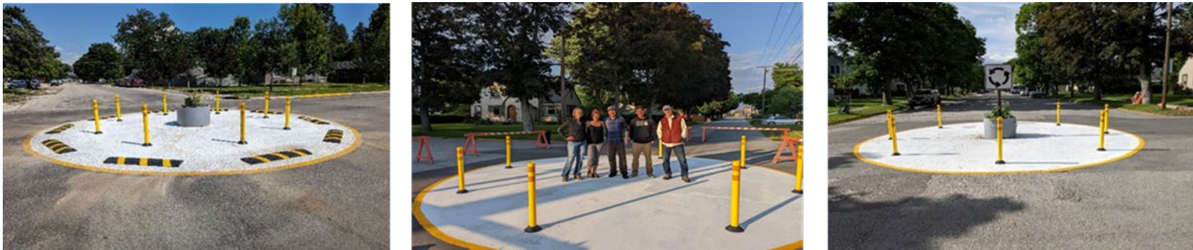
Figure 3: The pop-up traffic circles were completed (left, center, right) through the hard work of the installation crew (center).
