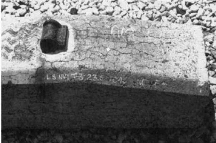
Figure 1.19 Cracking of prestressed concrete tie due to delayed ettringite formation (Hime, 1996)
