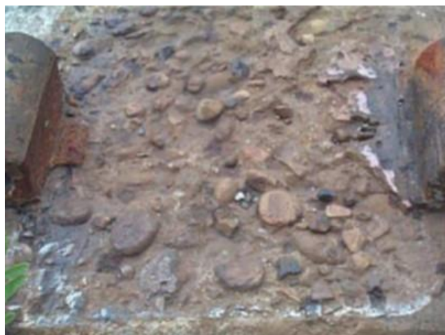
Figure 1.15 Rail-seat abrasion failure (Zeman et al., 2009)
