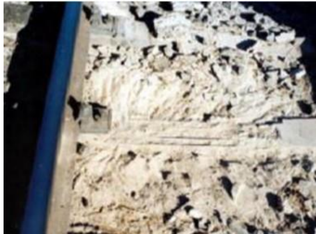
Figure 1.21 Failure of concrete tie as result of bar corrosion (Mohammadzadeh and Vahabi, 2011).
