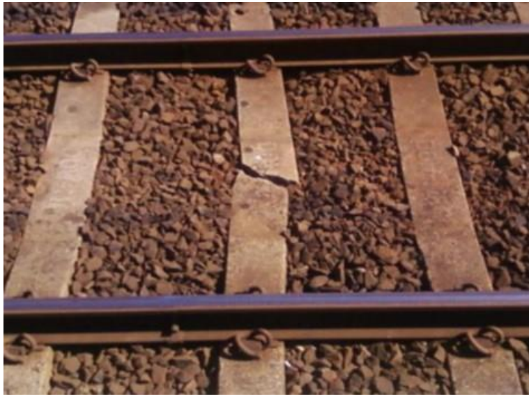
Figure 1.14 Flexural failure of PC tie due to negative bending (UK railway forums/broken tie, 2014)
