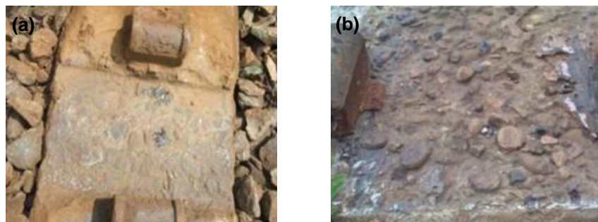
Figure 5.1 Prestressed concrete rail seat abrasion (a) Reiff et al. (2012), (b) Zeman et al. (2009)
