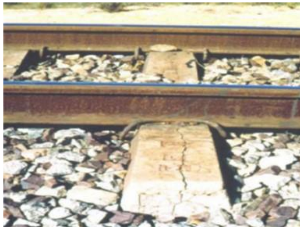
Figure 1.20 Cracking in concrete tie due to alkali aggregate reaction (Fournier et al., 2004)
