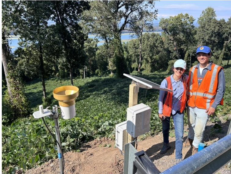
Figure 12: Photo of the finished monitoring station at SR-35 near Section, AL. The rain gauge and cellular antenna are shown on the left, while the datalogger housing and solar panel are shown on the right with the graduate students from Auburn.
