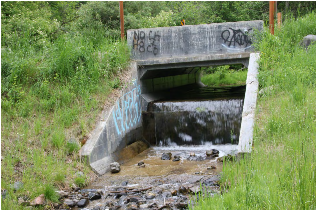
Figure 45 Aquatic Passage Assessment: The picture shows a culvert designed as a fish barrier
