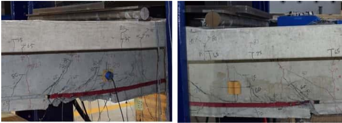
Figure 7-3 Inclined shear cracks near hook ends and interface failure for Specimen TB.G.H.P.01
