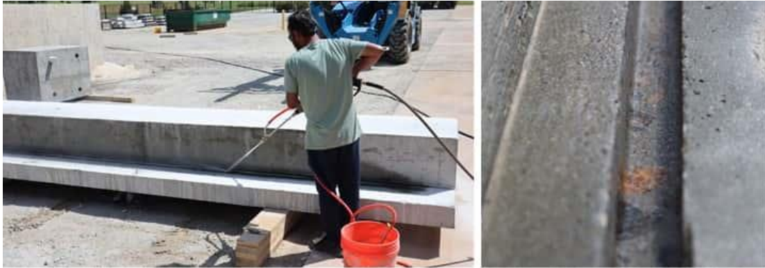
Figure 6-13 Low-pressure water blasting to clean the groove (Left) and Cleaned groove (Right)
