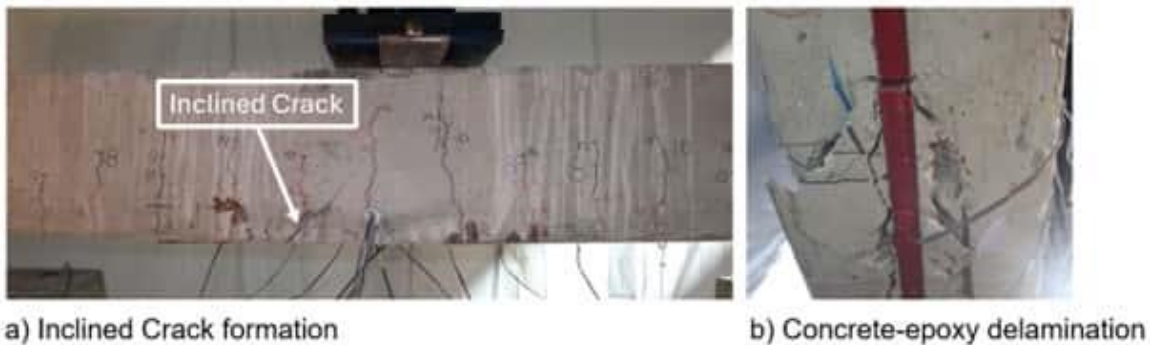
Figure 5-14 a) Inclined crack formation and b) concrete-epoxy interface delamination of SB40
