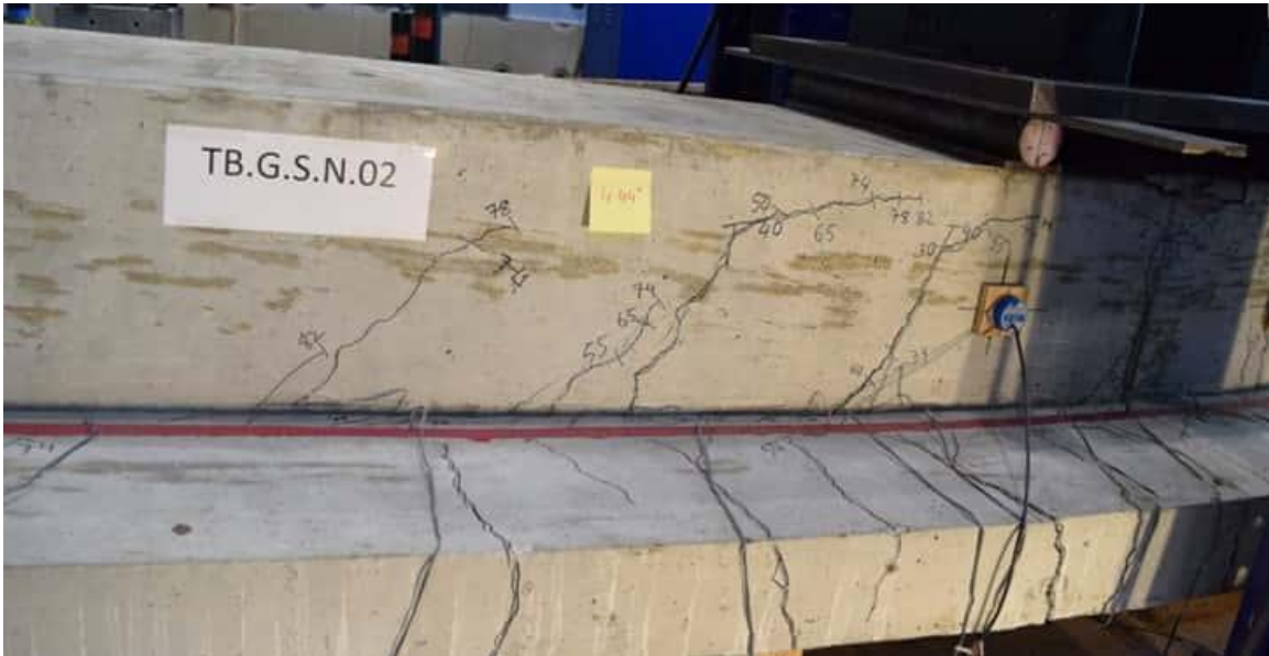
Figure 7-14 Concrete cracking pattern for Specimen TB.G.S.N.02 at 4.44 inches of mid-span displacement
