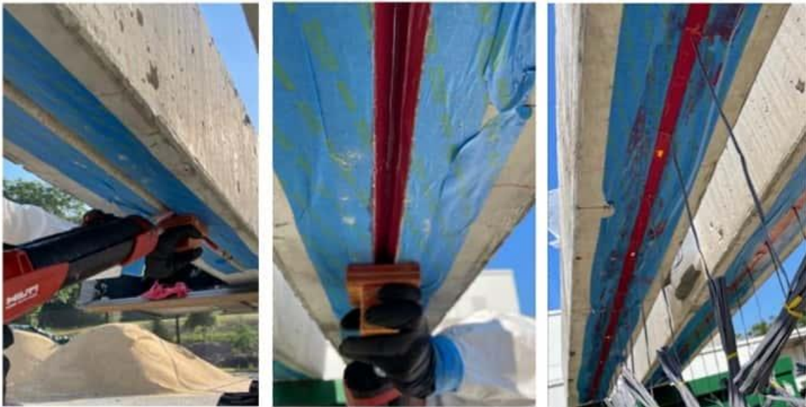
Figure 4-19 First lift of epoxy application (left and middle), and Installed TiAB after final epoxy lift (right)
