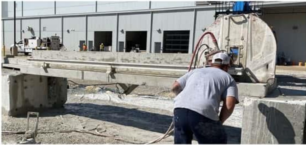
Figure 6-12 Cutting groove for positive bending test (Top) and for negative bending test (Bottom)
