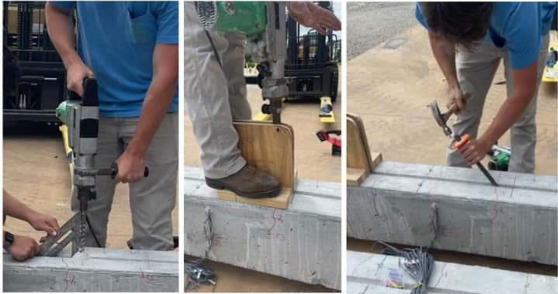
Figure 4-17 Hammer drill used for hole (left), beveling (middle), and chiseling to refine bevel
