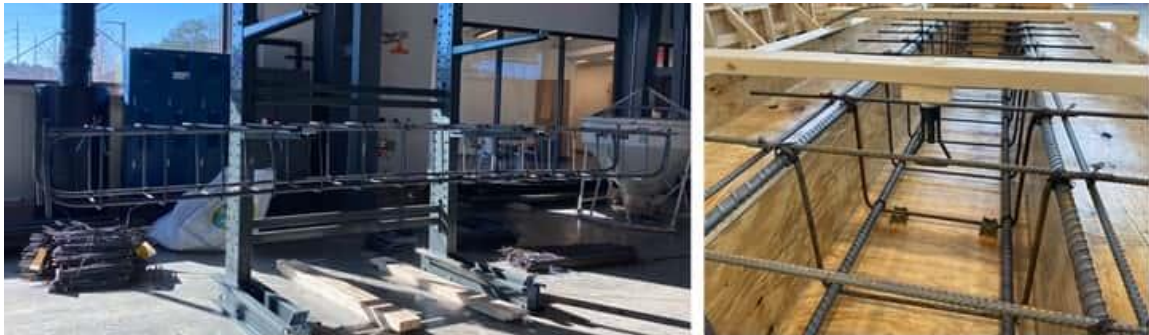
Figure 6-3 Rebar cage formation (Left) and formwork ready for casting with lifting device (Right)
