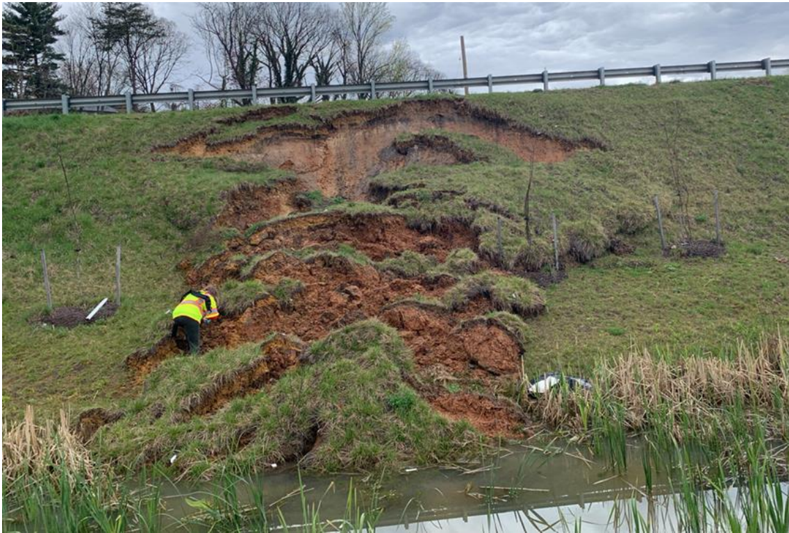
Figure 3.19. Landslide happened on April 4, 2024, at site 11.
