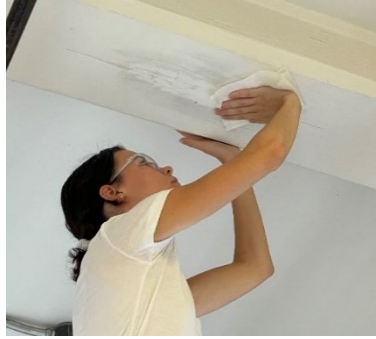
(c) Clean the substrate surface with acetone.
