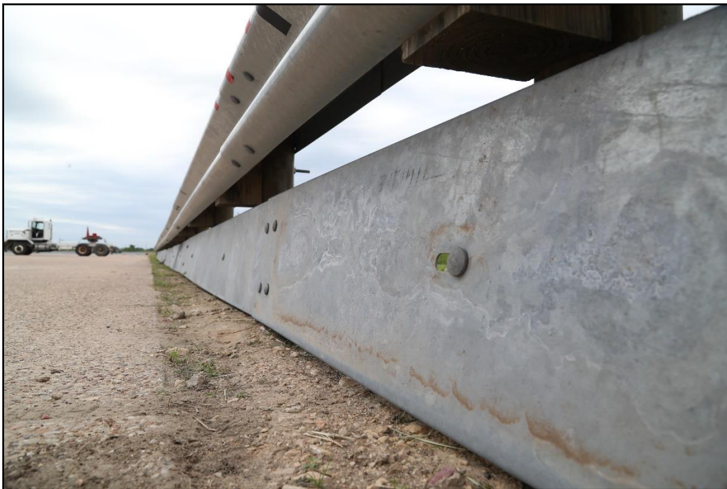
Figure 6.13. Enhanced Motorcycle Guard Fence System Rubrail Detail prior to Testing for 469943-01-1A, 469943-01-2, 469943-01-3, and 469943-01-4.
