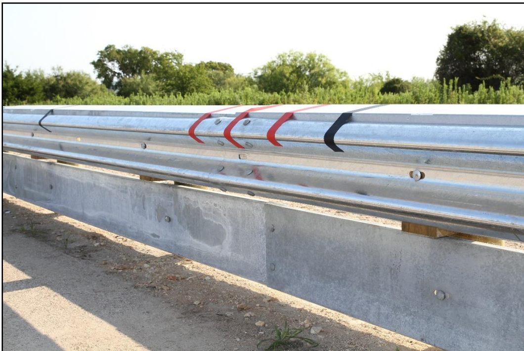
Figure 6.3. Enhanced Motorcycle Guard Fence System Rail Detail prior to Testing for 469940-03-1, 469940-03-2, 469940-03-3, and 469940-03-4A.
