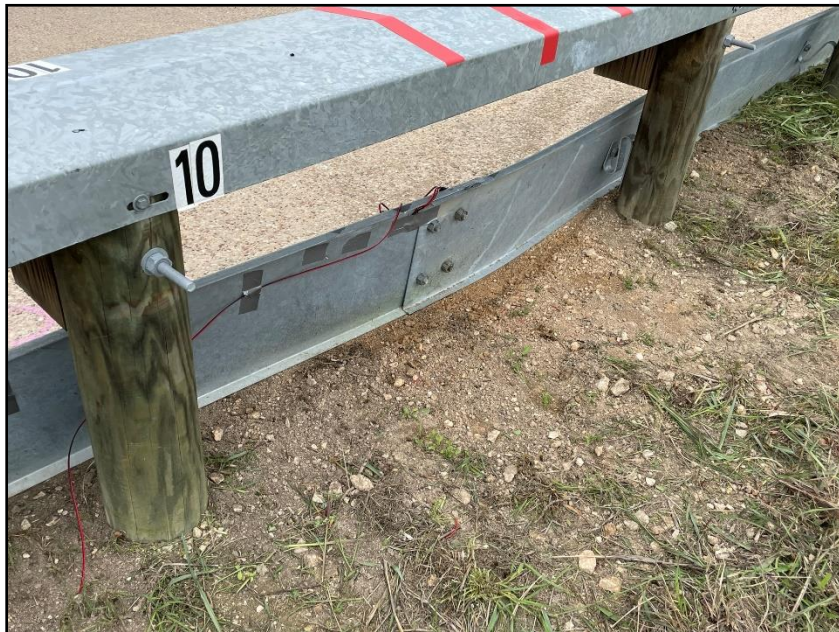
Figure 17.4. Field Side of the Enhanced Motorcycle Guard Fence System at Impact Location after Test 469943-01-2.
