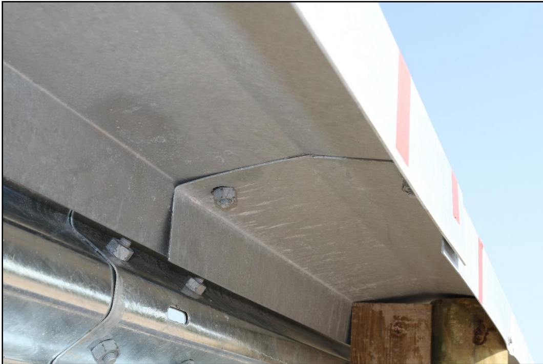
Figure 6.7. Enhanced Motorcycle Guard Fence System Cap Rail Hardware Detail prior to Testing for 469940-03-1, 469940-03-2, 469940-03-3, and 469940-03-4A.
