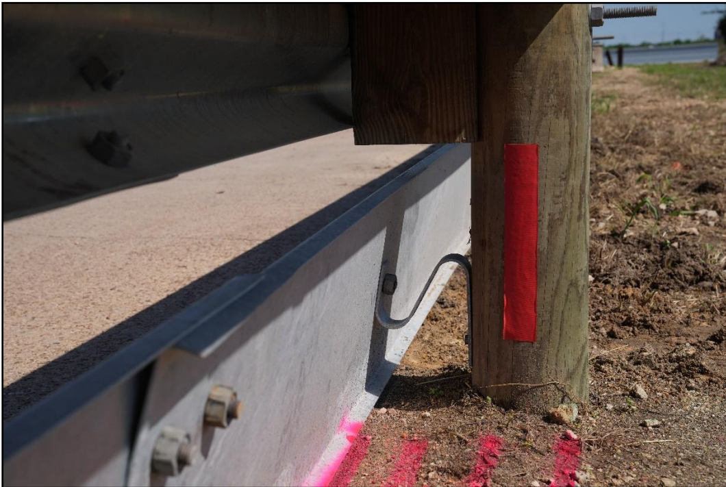
Figure 6.10. Enhanced Motorcycle Guard Fence System Rubrail Bracket Detail prior to Testing for 469942-01-1.
