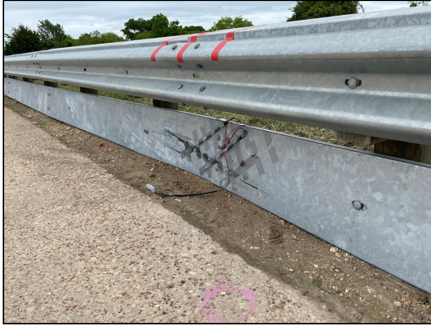
Figure 17.3. Traffic Side of the Enhanced Motorcycle Guard Fence System at Impact Location after Test 469943-01-2.
