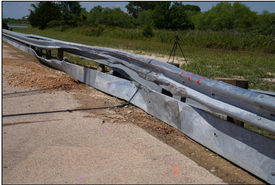
Figure 19.5. Traffic-Side View of the Enhanced Motorcycle Guard Fence System at Impact Location after Test 469943-01-4.
