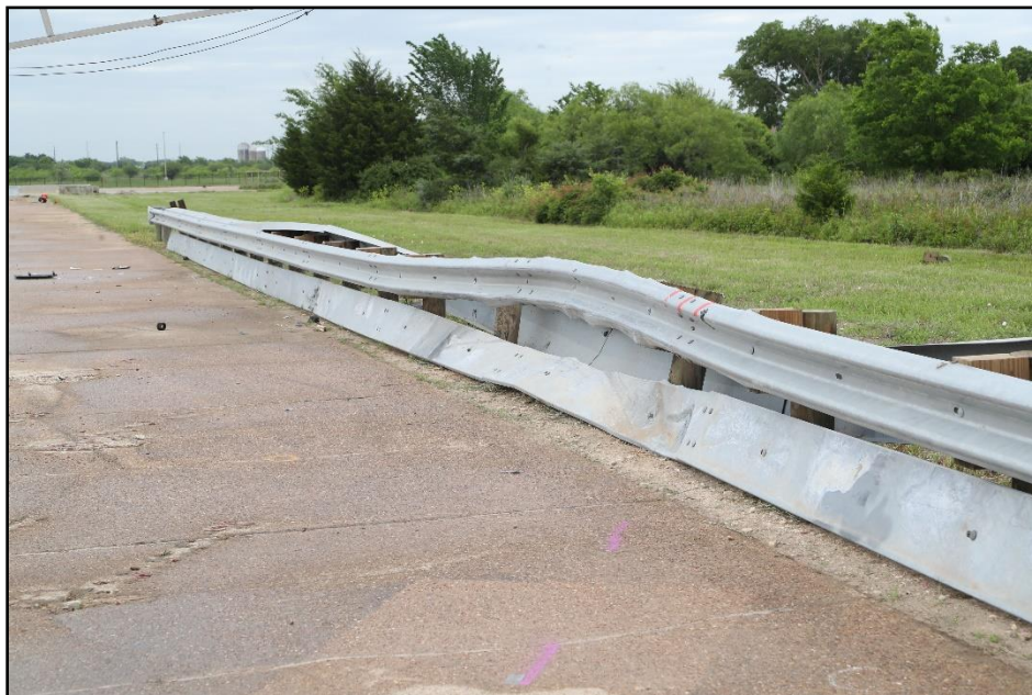
Figure 18.5. Traffic-Side View of the Enhanced Motorcycle Guard Fence System at Impact Location after Test 469943-01-3.
