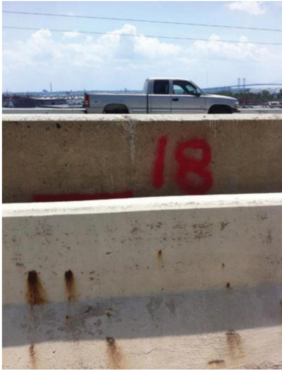
Figure 3-5 Settling Issue Between Northbound & Southbound Median Barriers (Benton, 2014)
