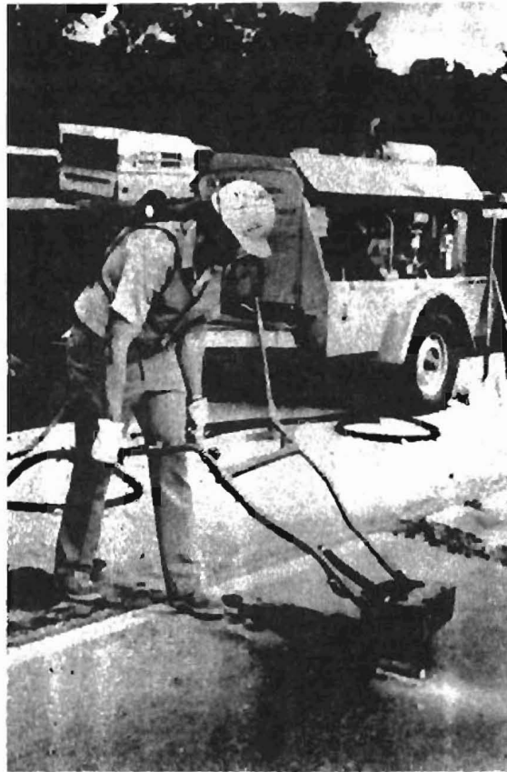
Fig. 4.10 Opening (Chasing) Cracks.
