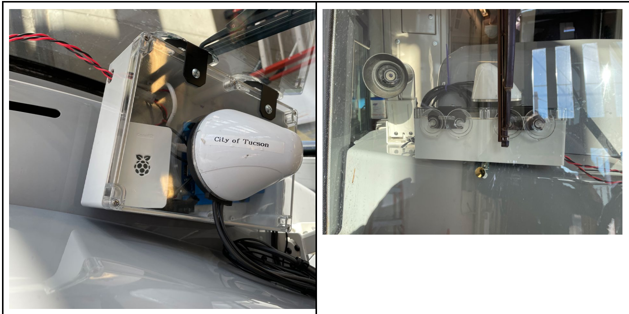
Figure 18: Streetcar OBU installation (based on Tucson Sunlink Streetcar installation)
