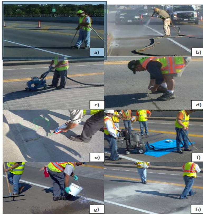
Figure 9. Typical Operations During Concrete Crack Sealing – a) blowing surface with air b) sand blasting c) shot blasting d) bottle application e) caulk gun application f) pump application g) flood application h) sand casting on surface (Oman, 2014)
