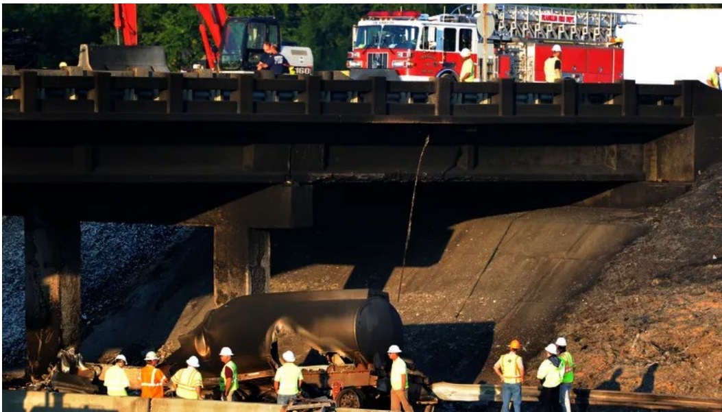
Figure 1.1 Truck explosion on I-65 at the Peytonsville Road bridge [1]
