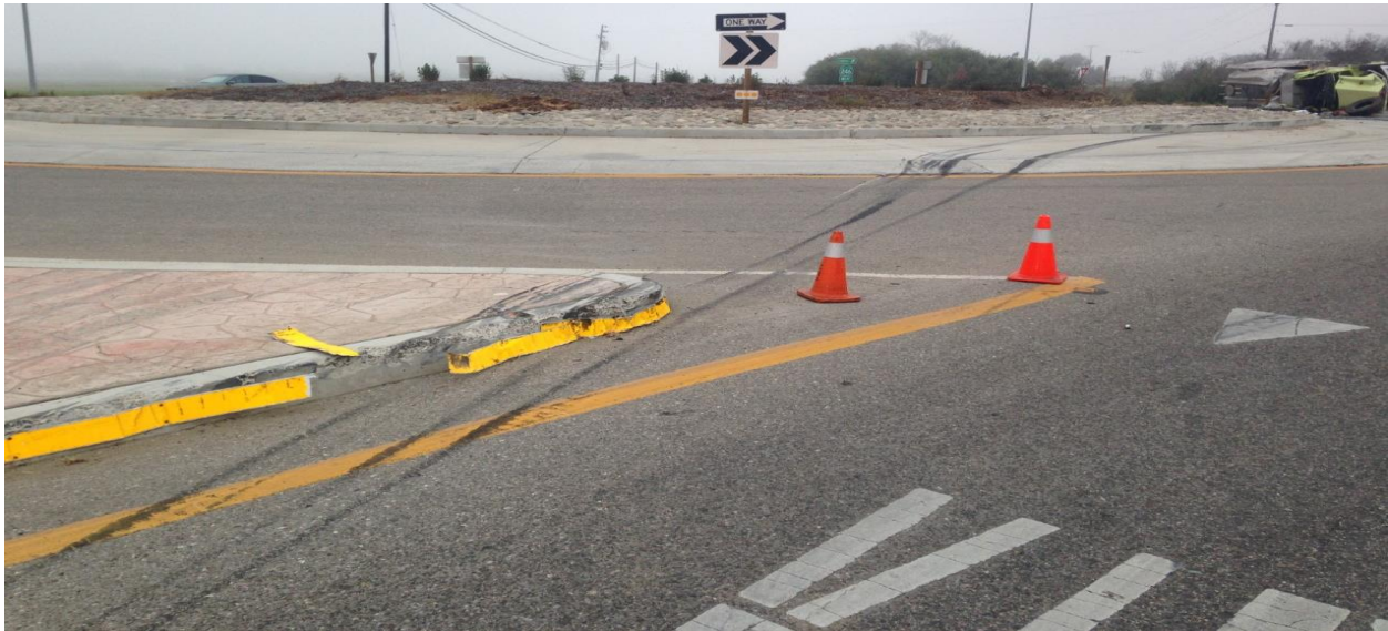
Figure A.8: A vehicle headed toward the roundabout, caused an accident despite the speed limitation. The splitter island was broken as the result. Image courtesy of Caltrans.
