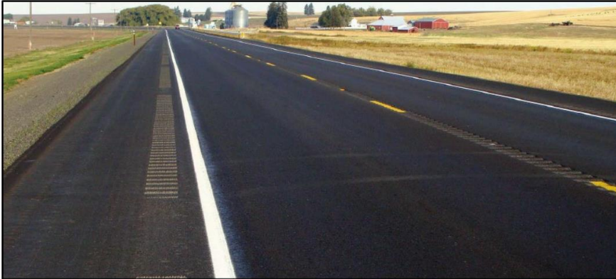
Image source: Guidelines for Installing Rumble Strips on California State Highways (https://dot.ca.gov/-/media/dot-media/programs/safety-programs/documents/policy/20-07-rumble-strips-guidelines-and-memo-011421-a11y.pdf)
