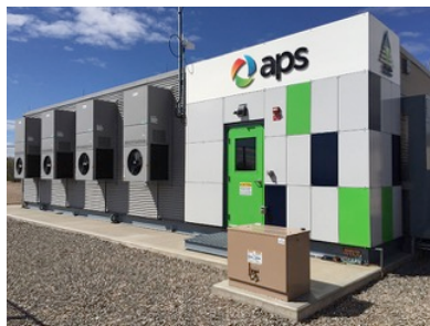
Figure 22. Arizona Public Service's 2-MW battery storage project in Surprise, Ariz., before a fire in April took it offline.
