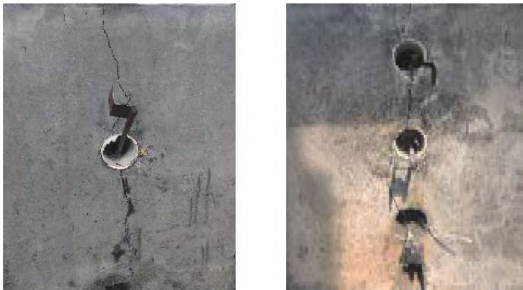
Figure 1.7 Specimen surface damage pattern (Xiao et al. 2022)
