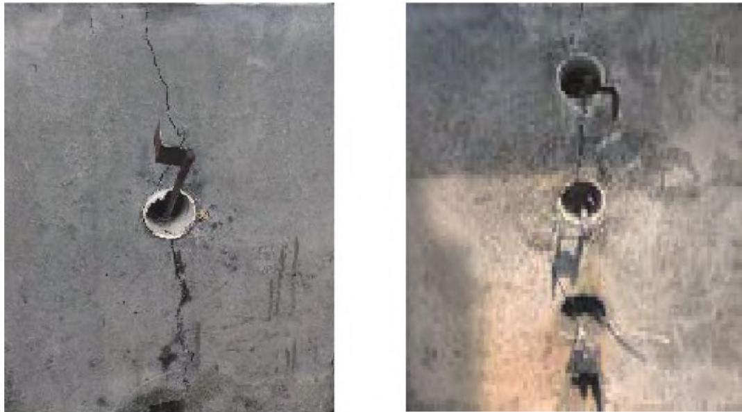
Figure 1.7 Specimen surface damage patterns (Xiao et al., 2022)
