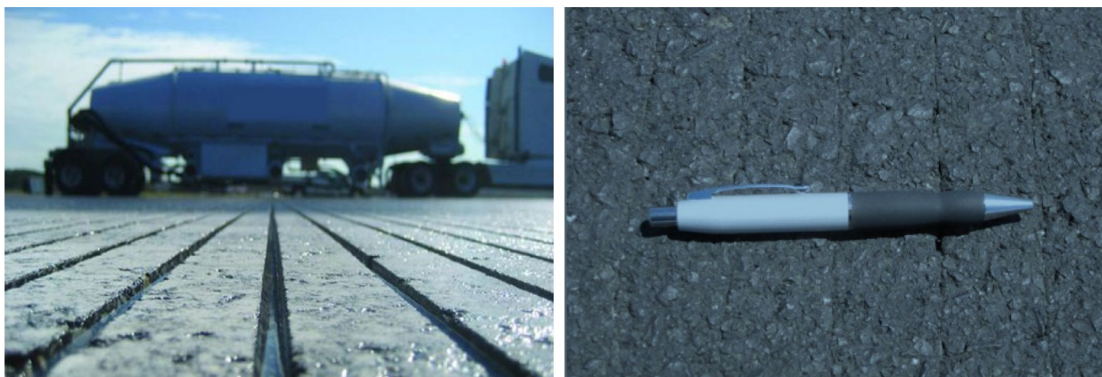
Figure 8. Runway grooves (left) and groove closure (right); a pen is included in the photograph on the right to show the closure of the grooves (Source: Jamieson and White, 2019).
