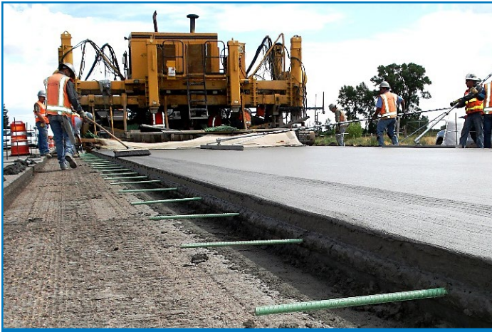
EDC-6 helped spread the word on concrete overlays with performance-engineered mixtures and new design procedures that improve durability and performance.
