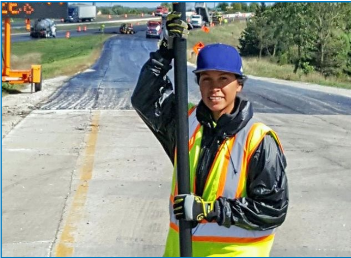
Tia Menore is one of a growing number of success stories emerging from Wisconsin DOT's Highway Construction Skills Training program.
