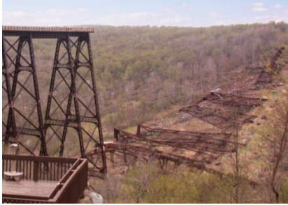
Figure 1.2 Kinzua bridge (F1 tornado in 2003)
