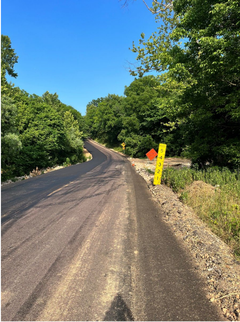
Figure 2.3 Area of periodic Flooding
