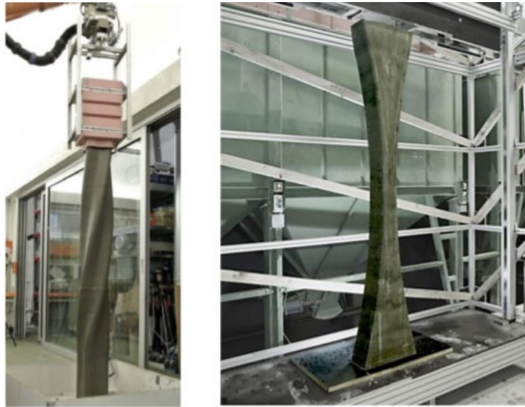
Figure 2.2 Smart Dynamic Casting System by ETH Zurich. (Asprone D., Auricchio F., et. al, 2018). [15].
