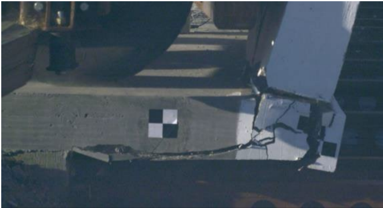
Figure 6.10 Damage in bridge deck supporting concrete parapet railing
