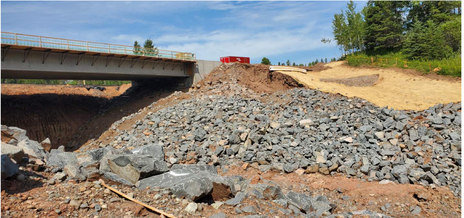
Figure 17. Recent slope failure along the the north bank of Deer Creek at Site 3. Headscarp visible near MN23.
