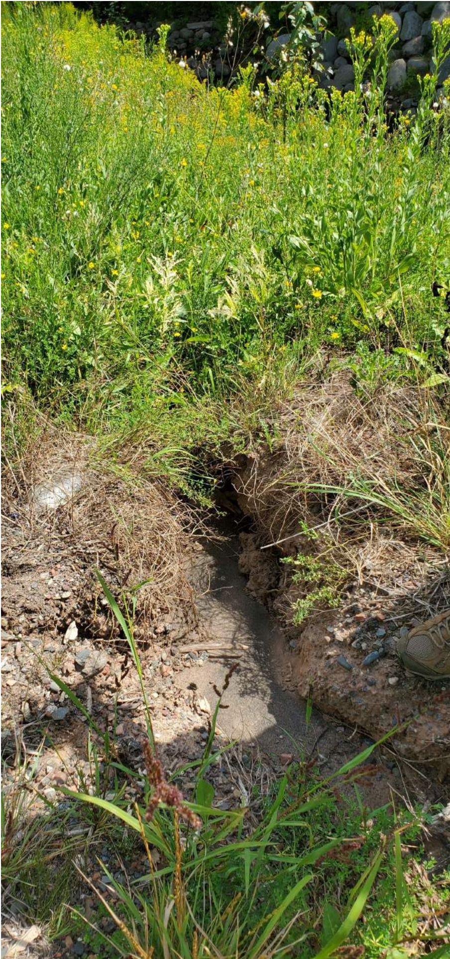
Figure 20. Small 1-ft deep channel formed near the exit of the culvert at Site 5.
