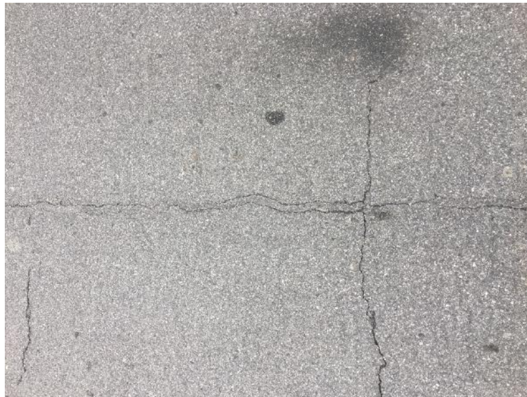
Figure 10. Cracking along routed and sealed cracks under micro surfacing.
