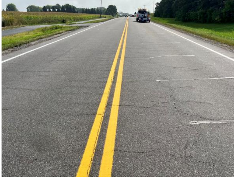
Figure 51. Overall condition of 70 th Street control section (thinlay only) after 4 years.
