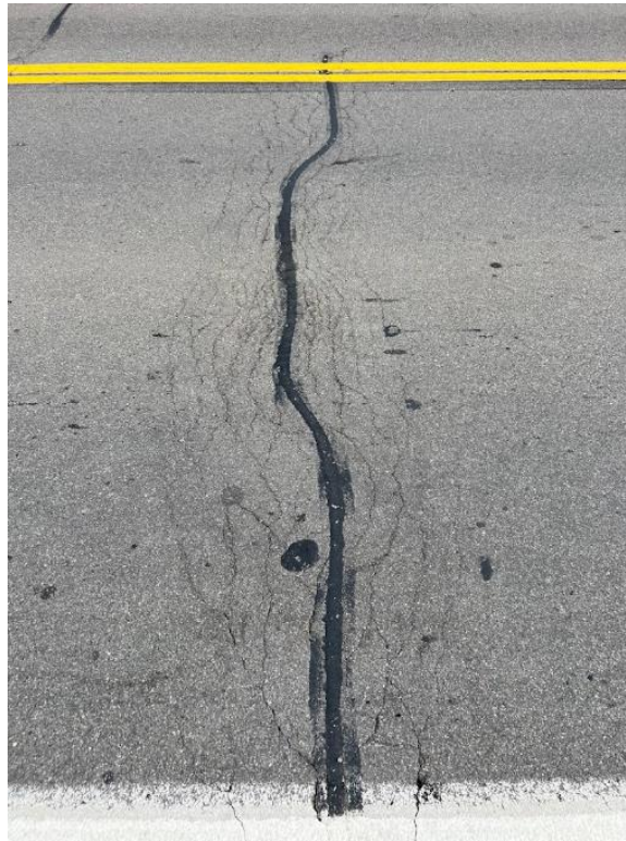
Figure 50. Transverse cracking in 70 th Street test section.
