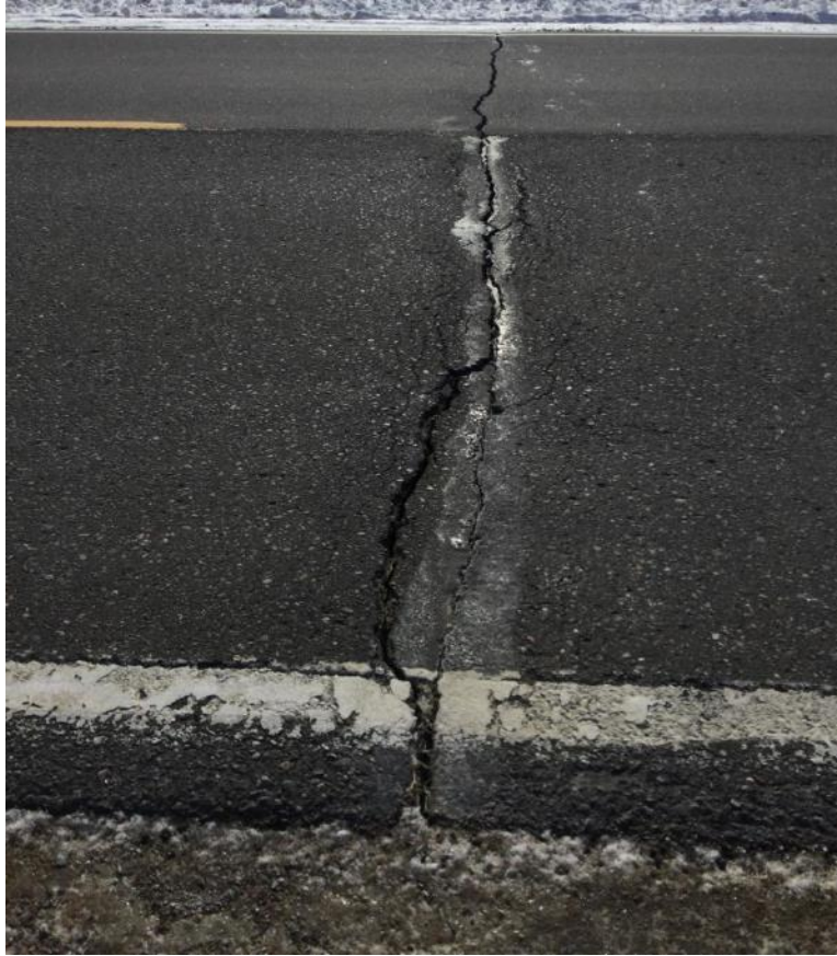
Figure 41. Severity of transverse cracking in treated and untreated sections.
