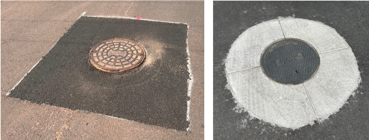
Figure 8. Example of square cut with asphalt collar (prior to paving the surface course) and round cut with concrete collar, after paving the surface course (courtesy NCE).
