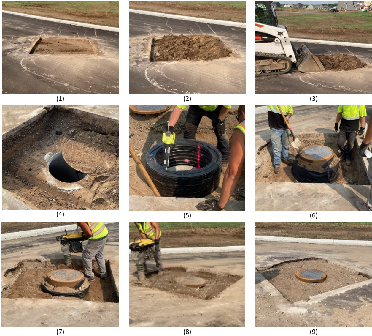
Figure 12. Unbound materials compaction sequence as part of utility cover adjustment (courtesy City of Woodbury, MN).
