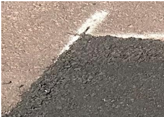
Figure 9. Example of sawcut overrun into adjacent pavement (square patch) (courtesy NCE).
