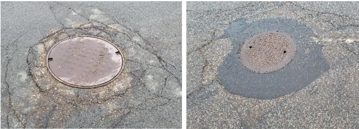
Figure 7. Pavement distresses around utility structure covers in Minnesota (courtesy NCE).
