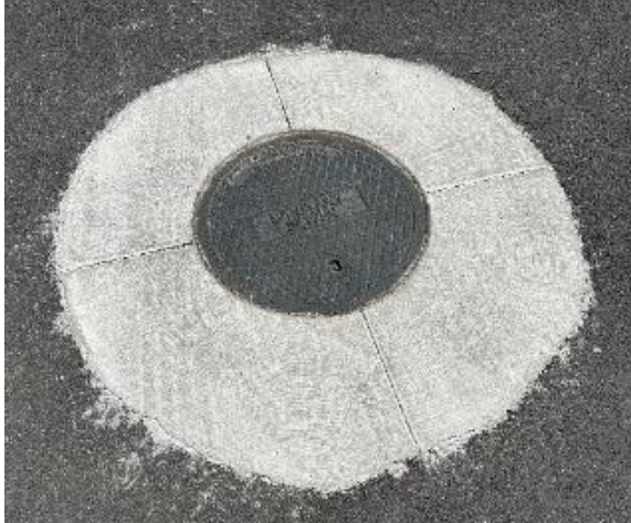
Figure 2. Example concrete collar scored at quarter points to initiate cracking (AzMAG detail) (courtesy NCE).
