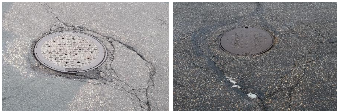
Figure 1. Examples of common pavement distresses around utility covers (courtesy NCE).
