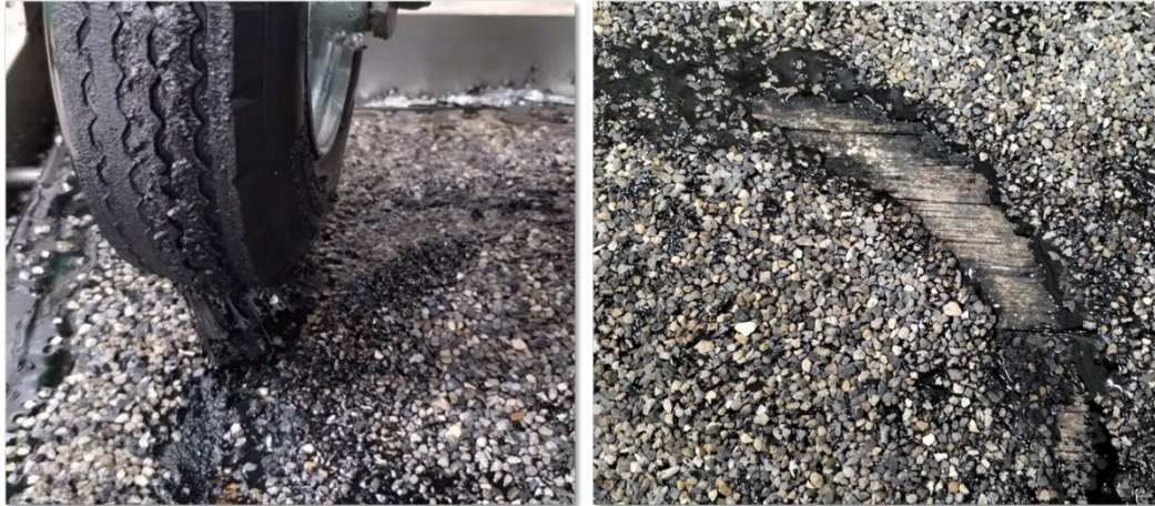
Figure 7.11 Severe bleeding and rutting in Emulsion CRS-2P slab after 30K polishing
