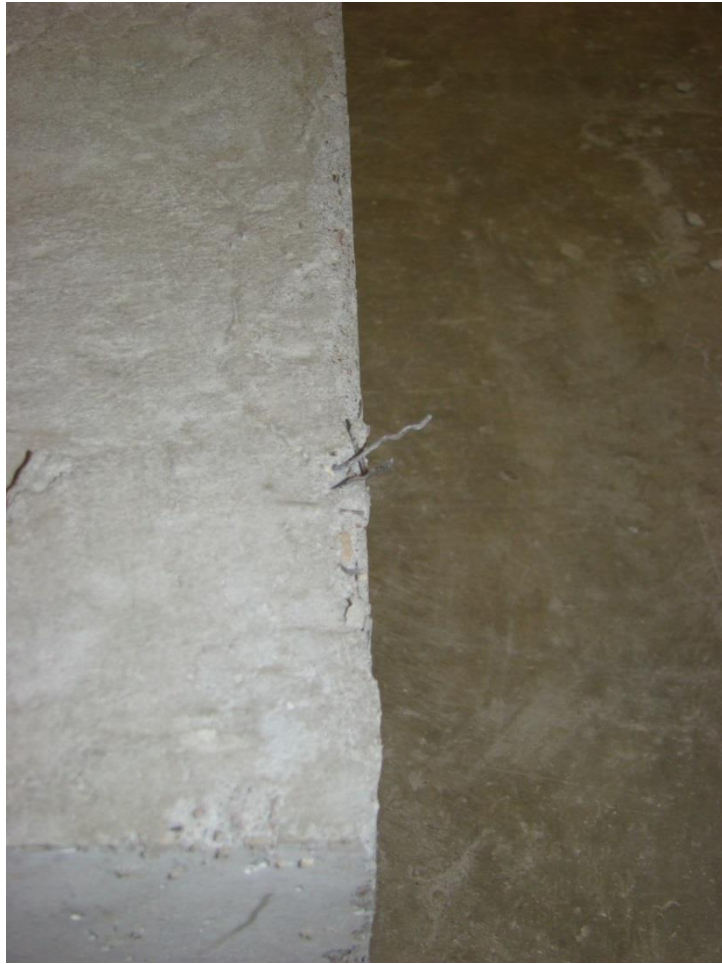
Figure 9-27: Steel fibers sticking out of the concrete surface
