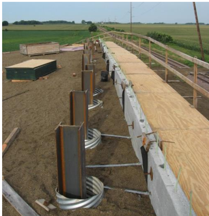
Abutment Piles in a Straight Line
