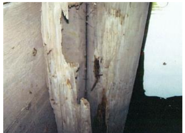
Figure 3-1f: Rot on third pile from east - south backwall prior to replacement.
