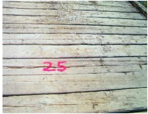
Figure 3-1h: Crack in 25th plank from north prior to replacement.
