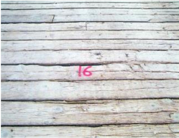
Figure 3-1g: Crack in 16th plank from north prior to replacement.
