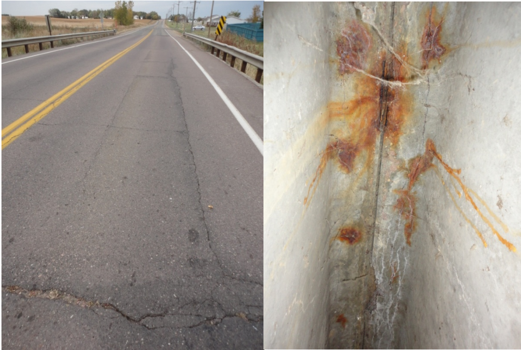
Figure 6-5: Leaking joints and spalling of concrete
