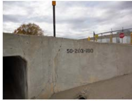
Cracking in the Wing Walls
