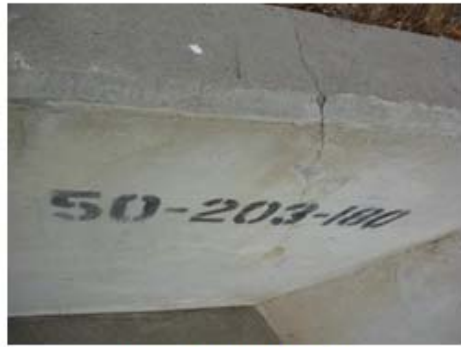
Crack through the Wall Thickness
