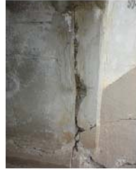
Cracking between the Culvert Wall and the Wing Wall Extension
