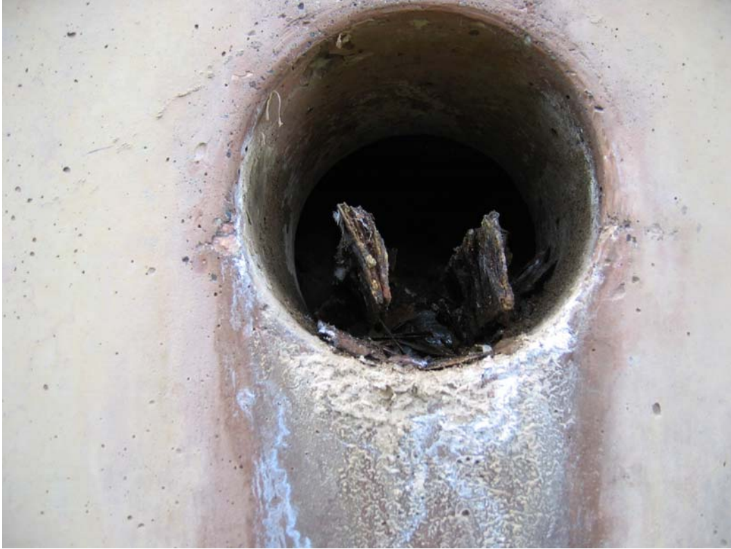
Figure 5 Severe corrosion of steel reinforcement straps in test location on Deadwood wall
