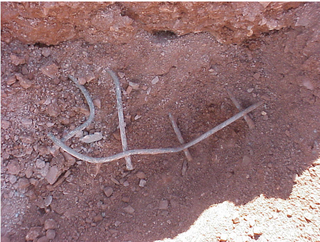
Figure 11 Mesh at station 25+89 EB lane showing severe deformation
