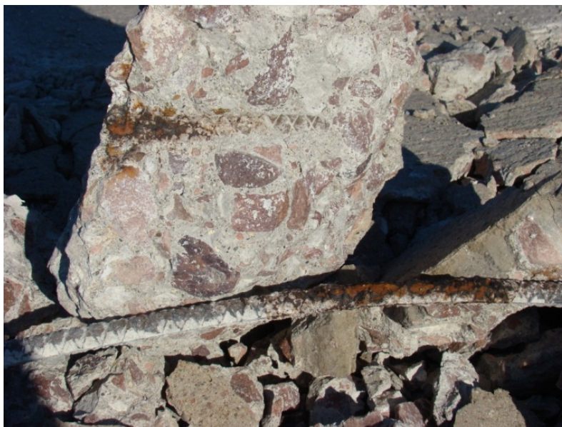
Figure 6-23: Localized corrosion found in the concrete rubble that was eventually removed
