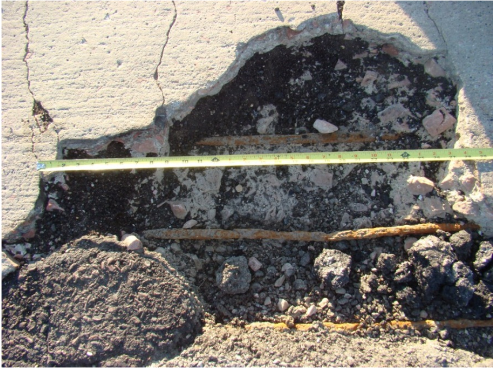
Figure 4-3: Corroded reinforcement exposed during CRCP removal
