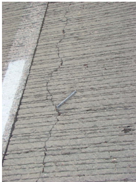
Figure 6-27: Longitudinal cracking on I-90
