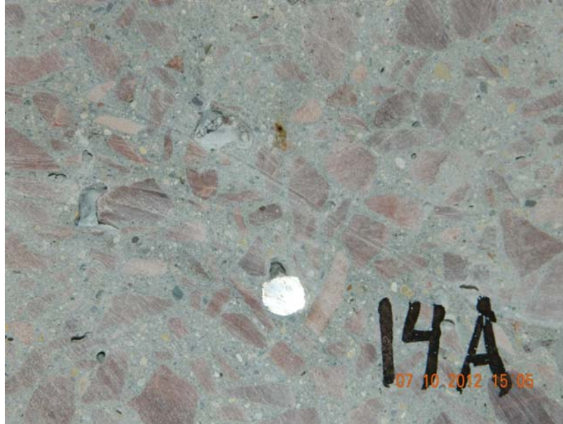
Figure 6-86: Saw cut along the crack of dry, cracked control specimen showing the reinforcement
