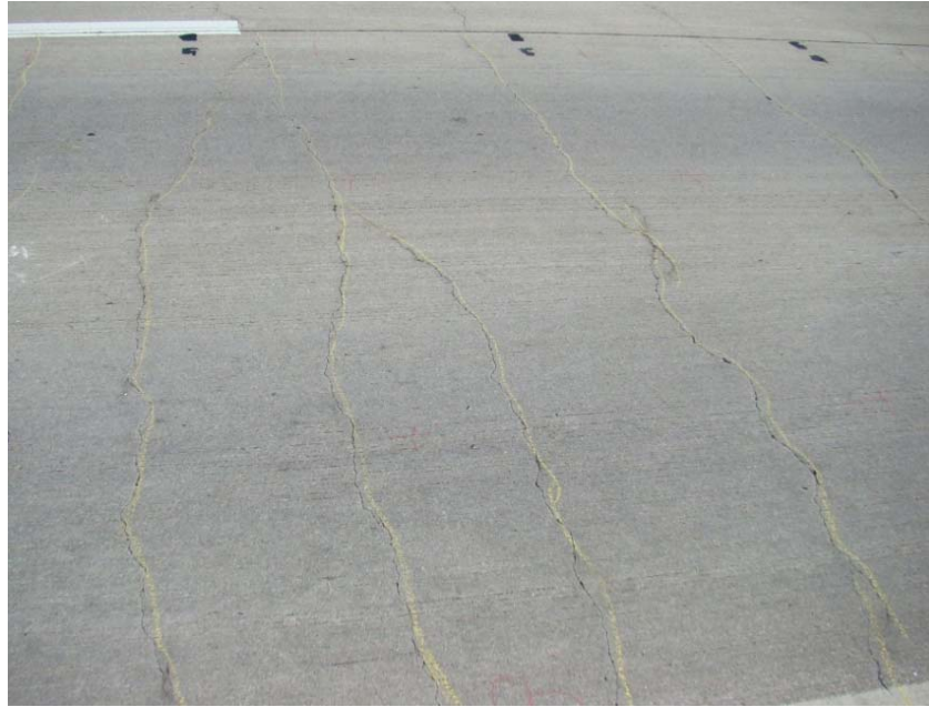
Figure 6-42: Cracking observed at MRM 168SB
