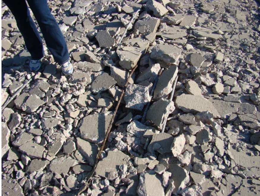
Figure 6-25: Corroded longitudinal reinforcing bar
