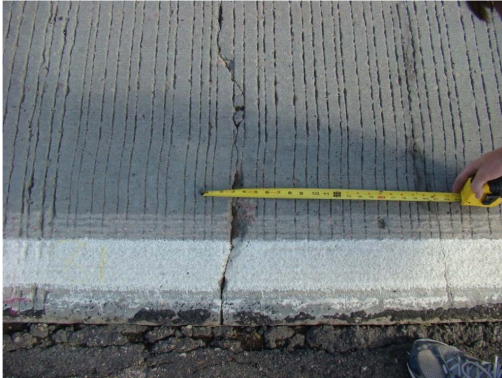
Figure 6-37: Wide crack exhibiting spalling at MRM 222
