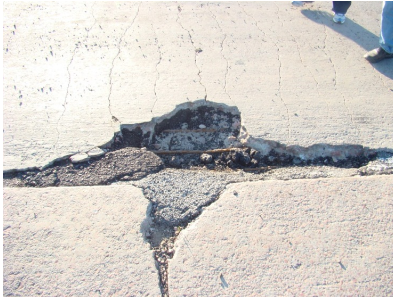
Figure 6-22: Patched pavement with exposed reinforcing steel
