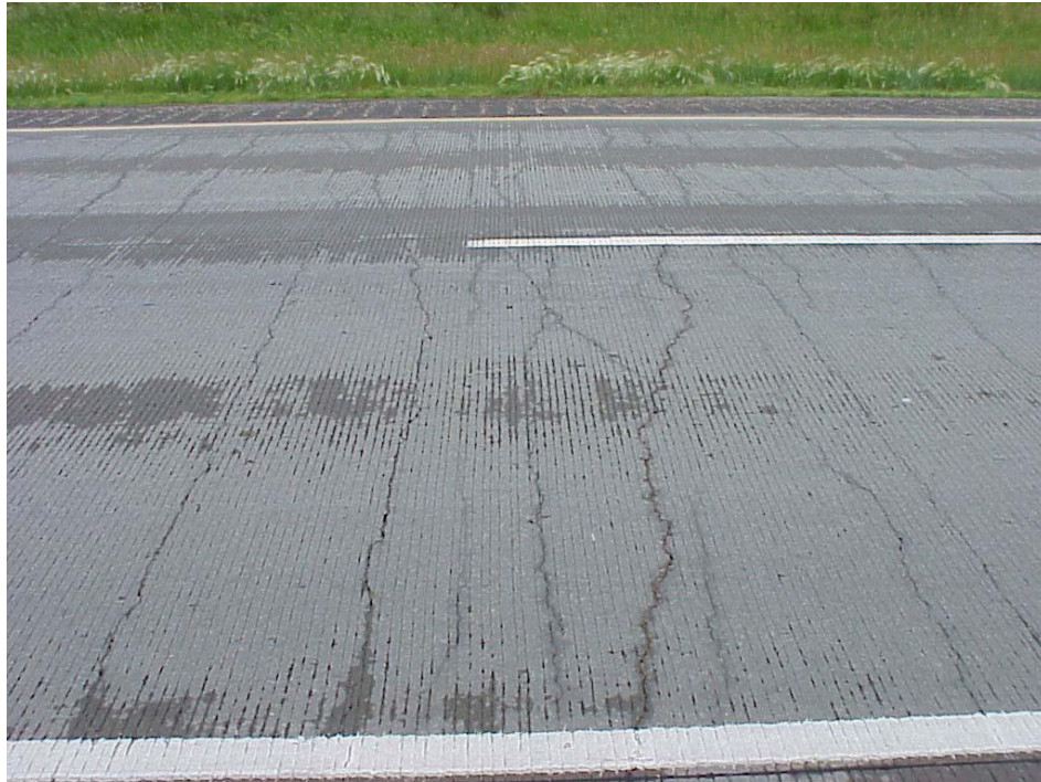
Figure 4-1: Network and Y-cracking (Johnston 2009)
