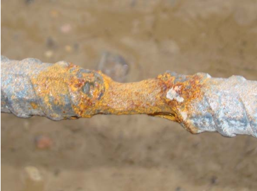
Figure 6-28: Severe loss of cross-sectional area
