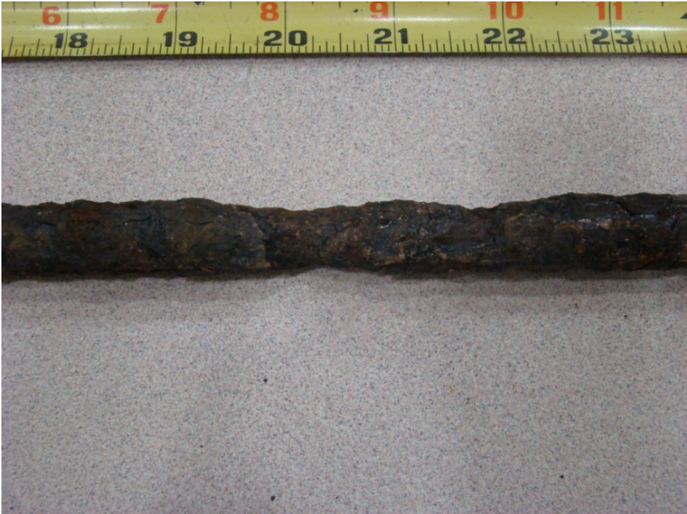
Figure 4-4: Corroded reinforcement removed from degraded CRCP
