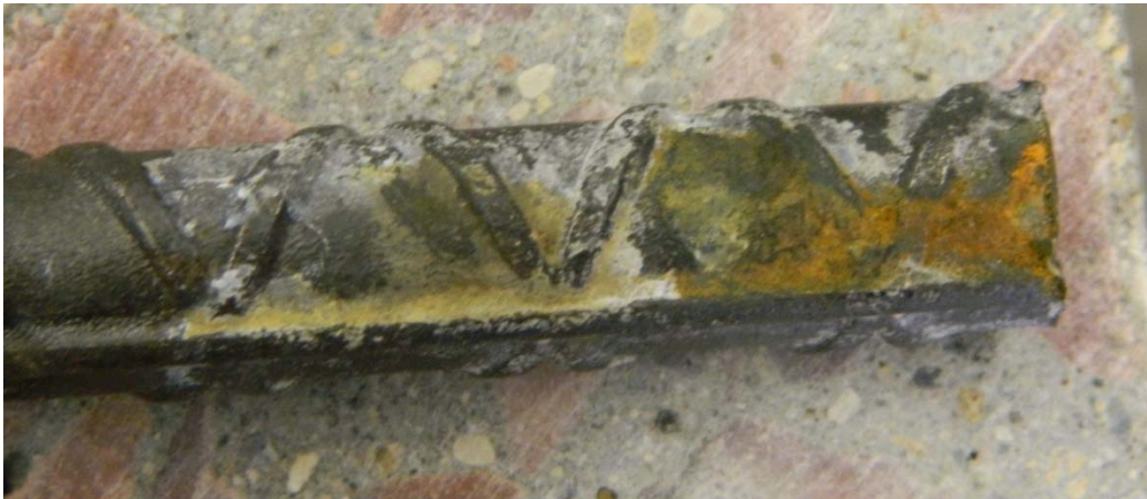
Figure 6-89: Close-up of corrosion of Specimen 16
