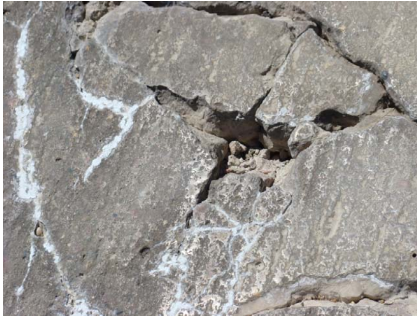
Figure 6-24: Spalled area with no signs of corrosion
