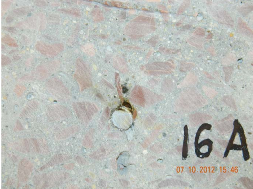
Figure 6-88: Saw Cut along the simulated crack of Specimen 16
