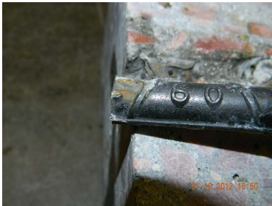
Figure 6-87: Close-up of corrosion of dry, cracked control specimen
