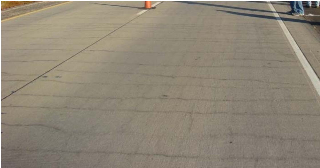
Figure 6-1: Cracking on Interstate 29 at MRM 87
