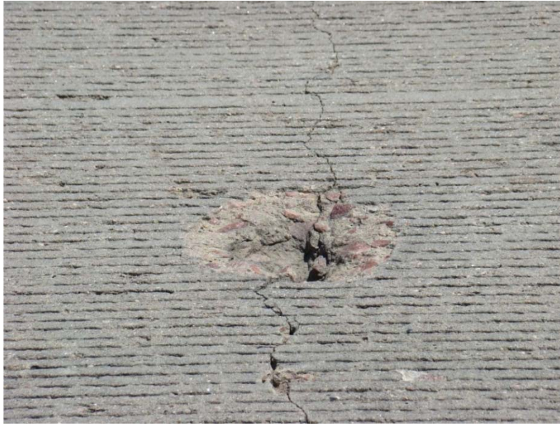
Figure 6-33: Spalling observed in passing lane at MRM 44
