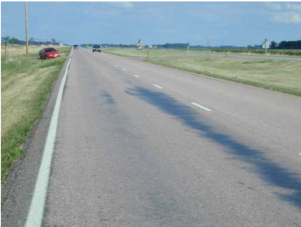
Figure A-8. Isolated area of bleeding before chip seal placement.
