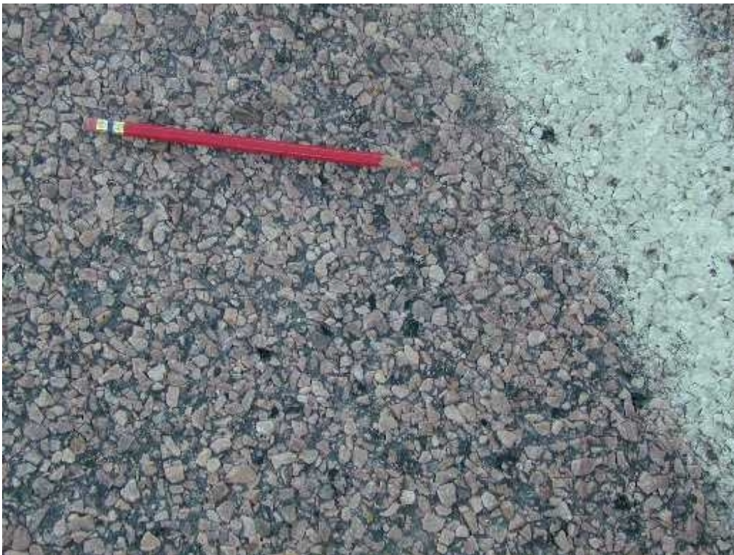
Figure A-26. Missing chips on SDDOT standard section with quartzite chips.
