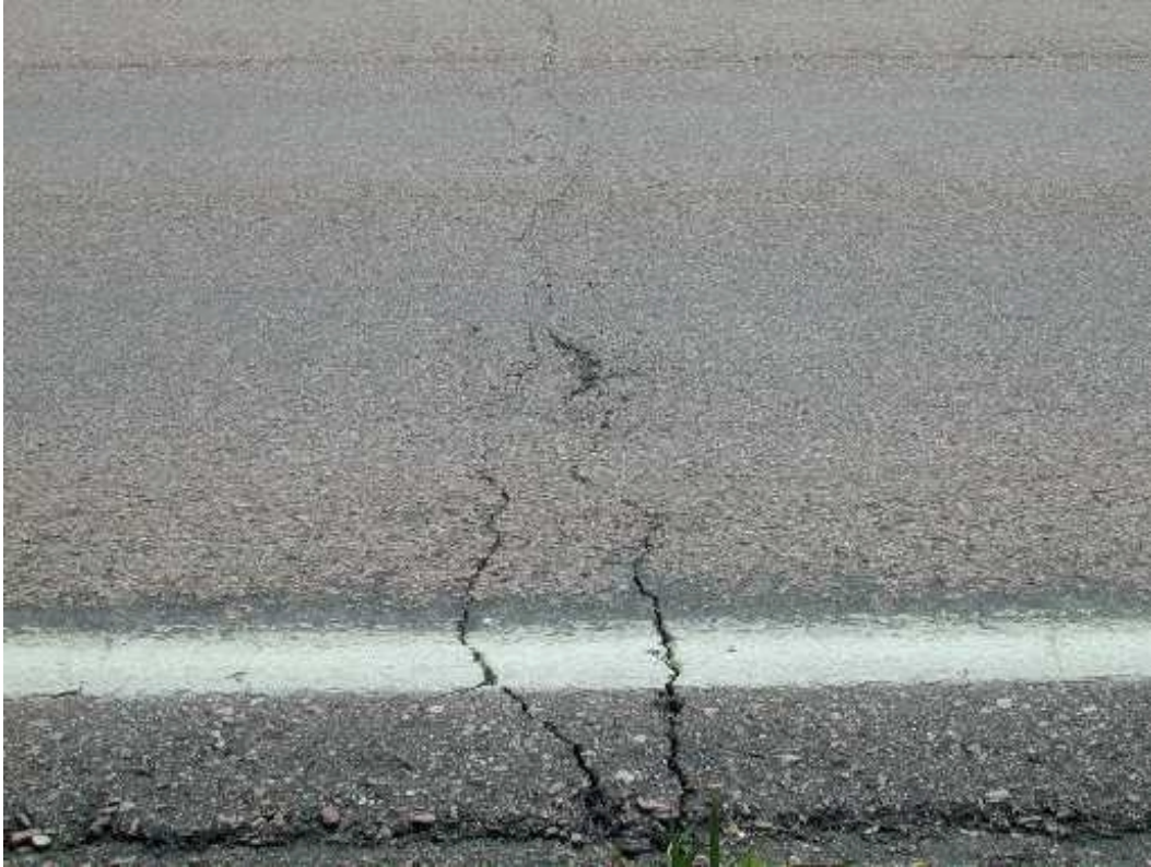
Figure A-7. Typical medium-severity transverse crack before chip seal placement.
