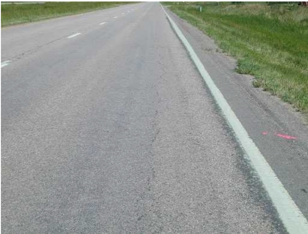
Figure A-6. Typical longitudinal crack before chip seal placement.
