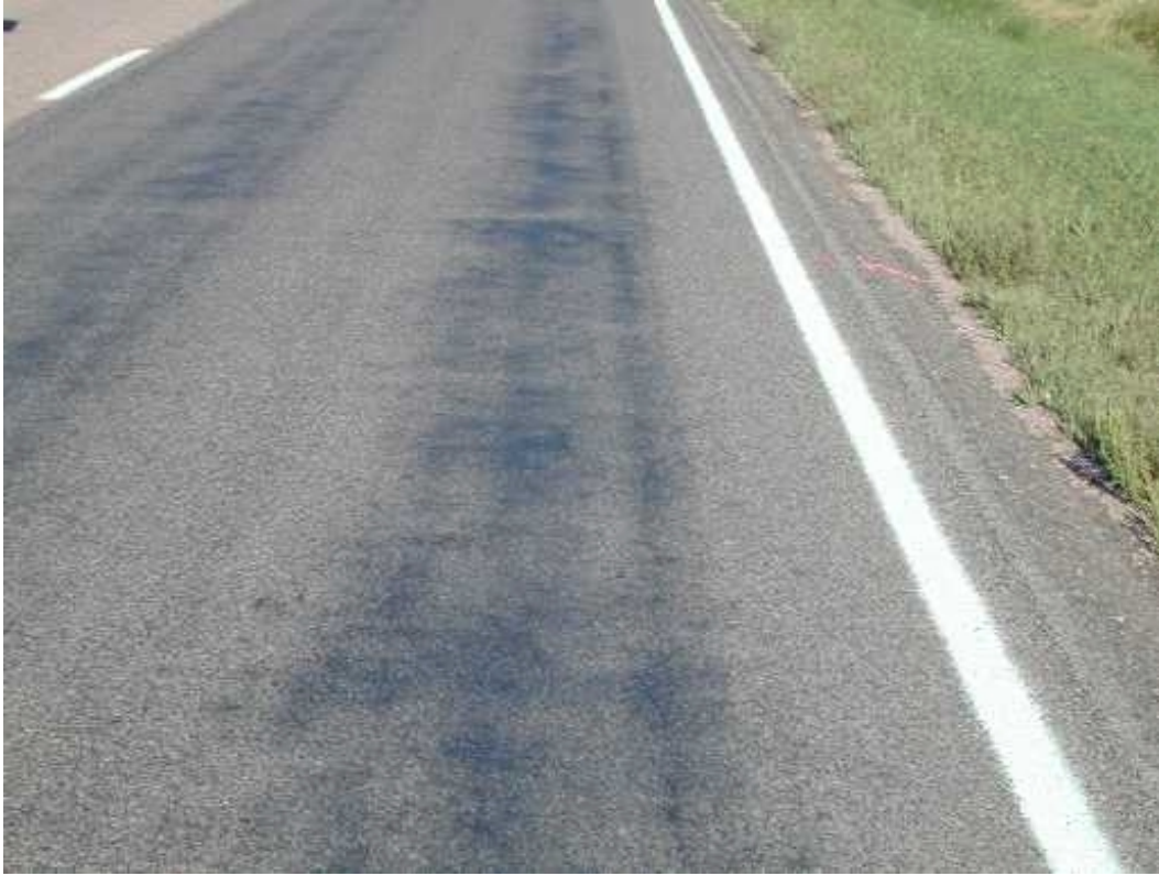
Figure A-27. Bleeding on choke stone section with quartzite aggregate.
