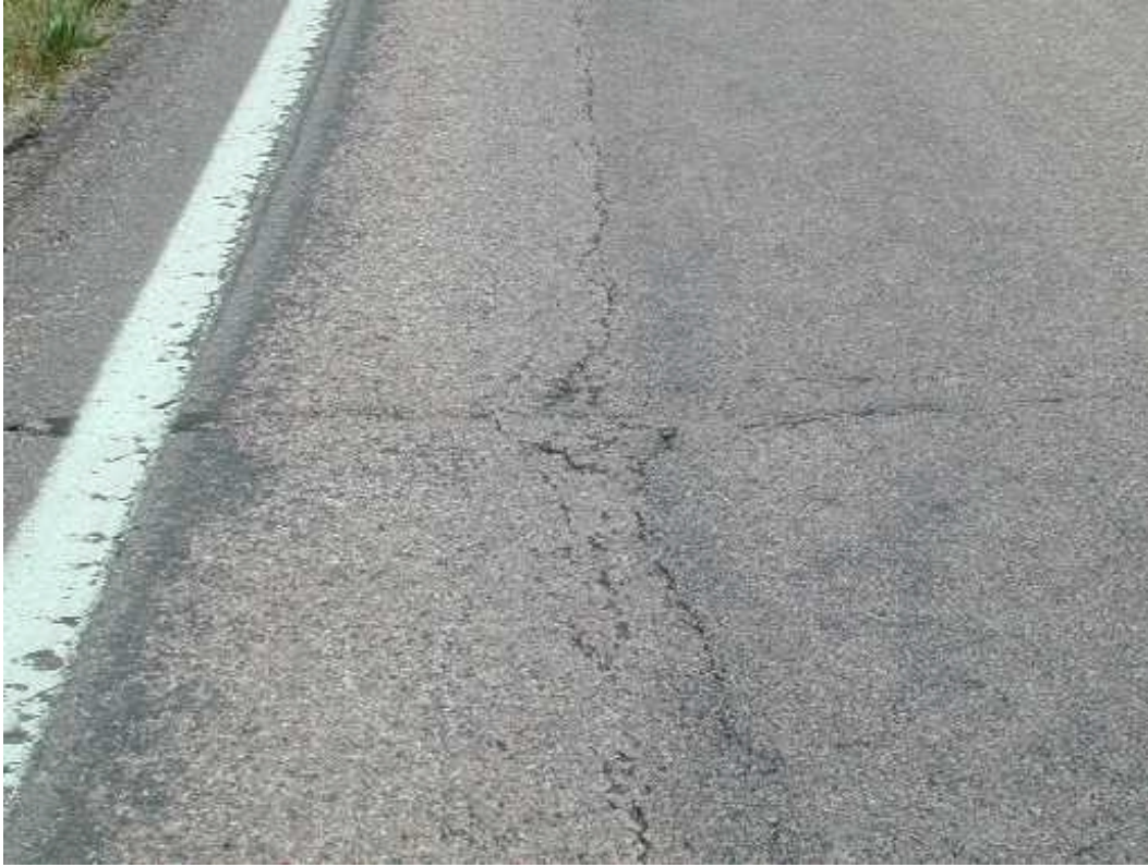
Figure A-5. Typical alligator cracking before chip seal placement.
