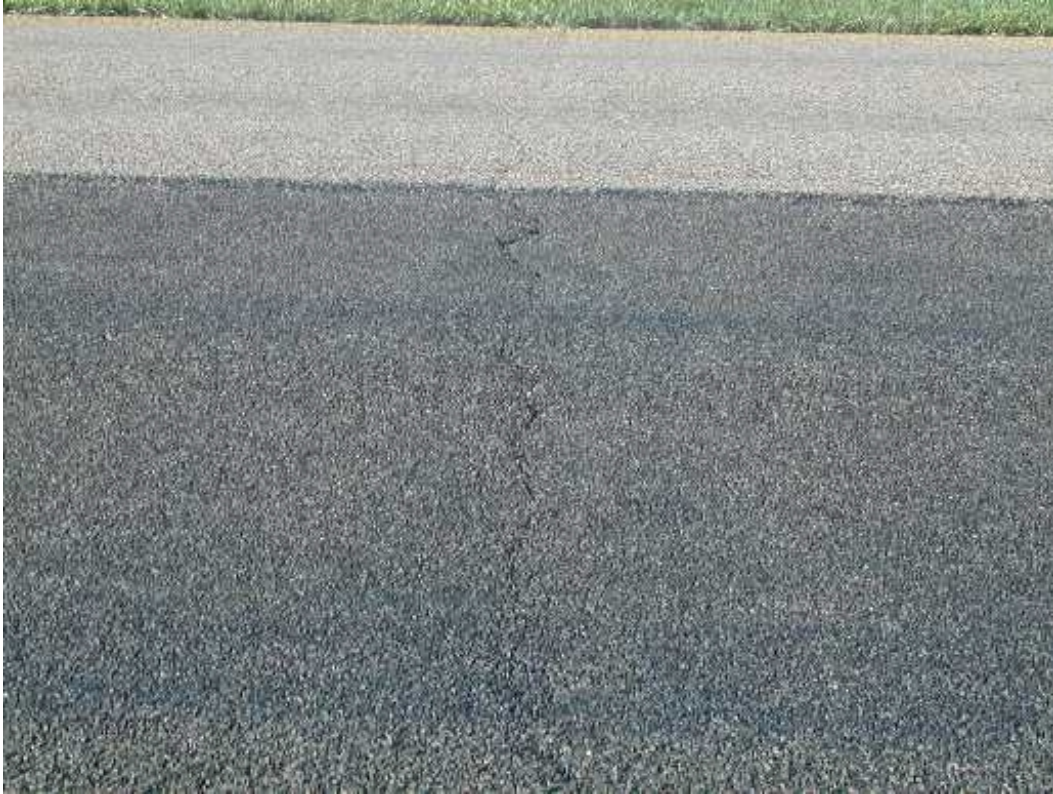
Figure A-25. Typical transverse reflective crack at 3-month follow-up.
