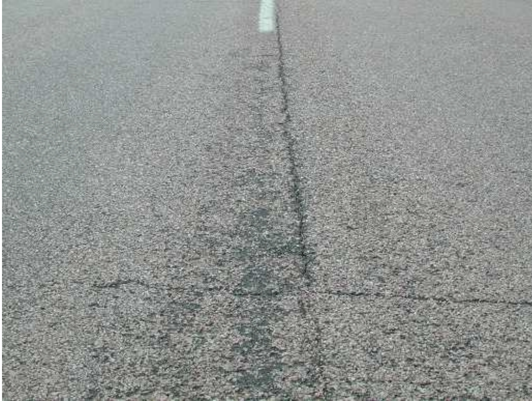
Figure A-3. Typical raveling along centerline before chip seal placement.
