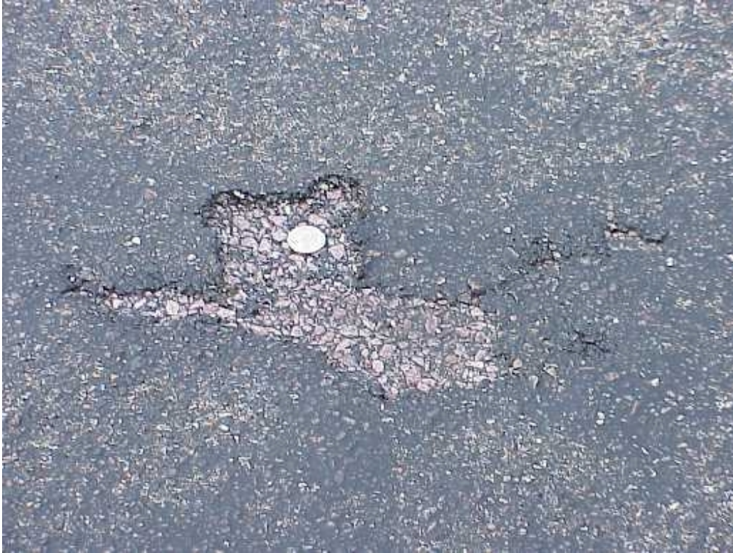
Figure A-29. Failed choke stone surface (natural aggregate) after 1 week.
