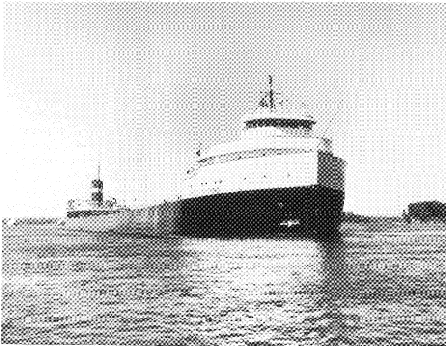
New 120-foot midbody (top) for Great Lakes ore carrier, WILLIAM CLAY FORD (bottom), is floated into dock at Fraser Shipyards, Superior, Wis., where it was fortified with steel beams and welded to bow and stern. Before she was cut in two, vessel was 647 feet long—already largest of five Ford Motor Co. carriers. Jumboizing permits WILLIAM CLAY FORD to carry additional 3,500 tons of taconite pellets each voyage she makes from Duluth, Minn., to Ford's Rouge steel operations in Dearborn, Mich.
