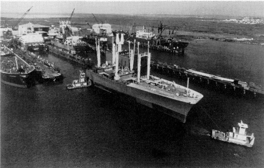
At Todd Shipyards in Galveston, Tex., tugs tow forward half of MORMACALTAIR out of dry dock so that new midbody of jumboized Moore McCormack general cargo ship can be floated in—and all sections connected.
