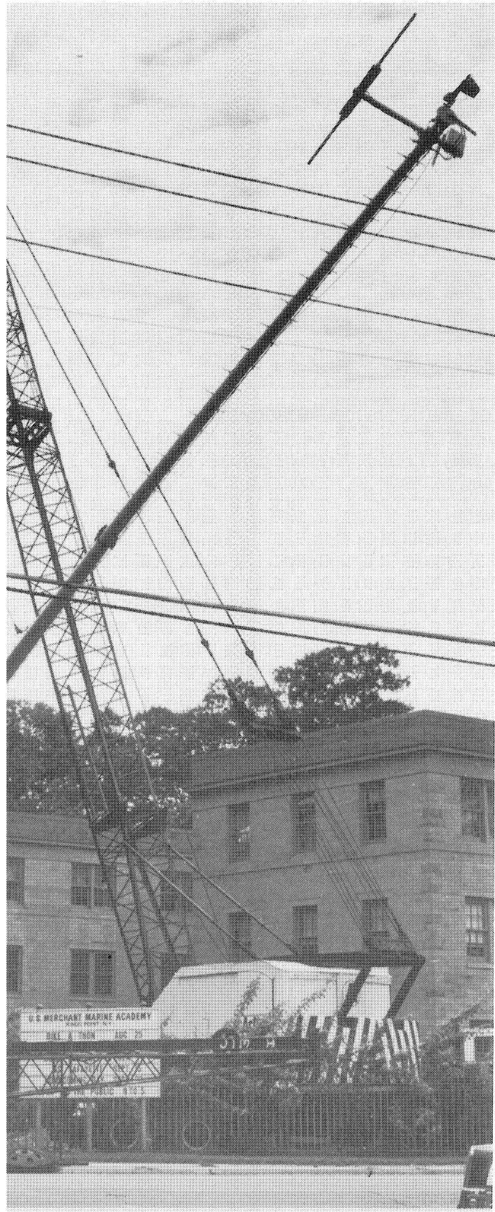
Erection of 180-foot mast with complex radar receiver mounted at top at National Maritime Research Center, Kings Point, N.Y. Radar unit monitors shipping in Long Island Sound as part of collision avoidance research project
