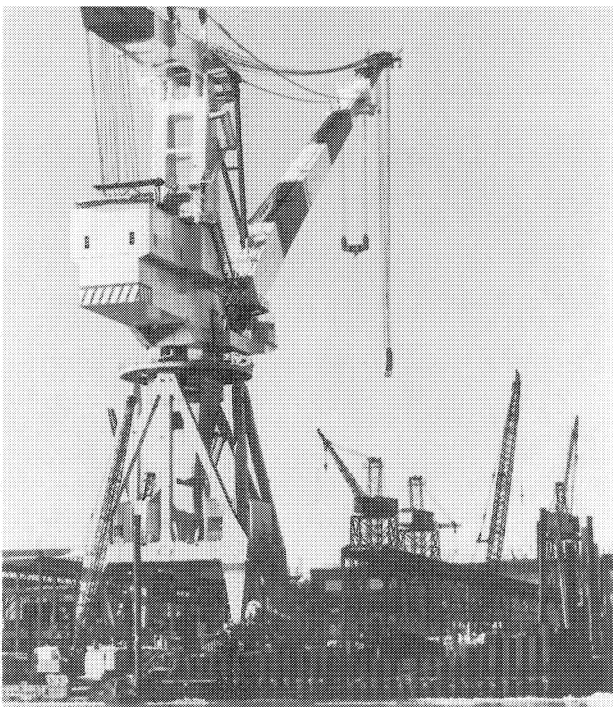
As part of modernization and expansion program, Bath Iron Works installed new 200-ton crane
