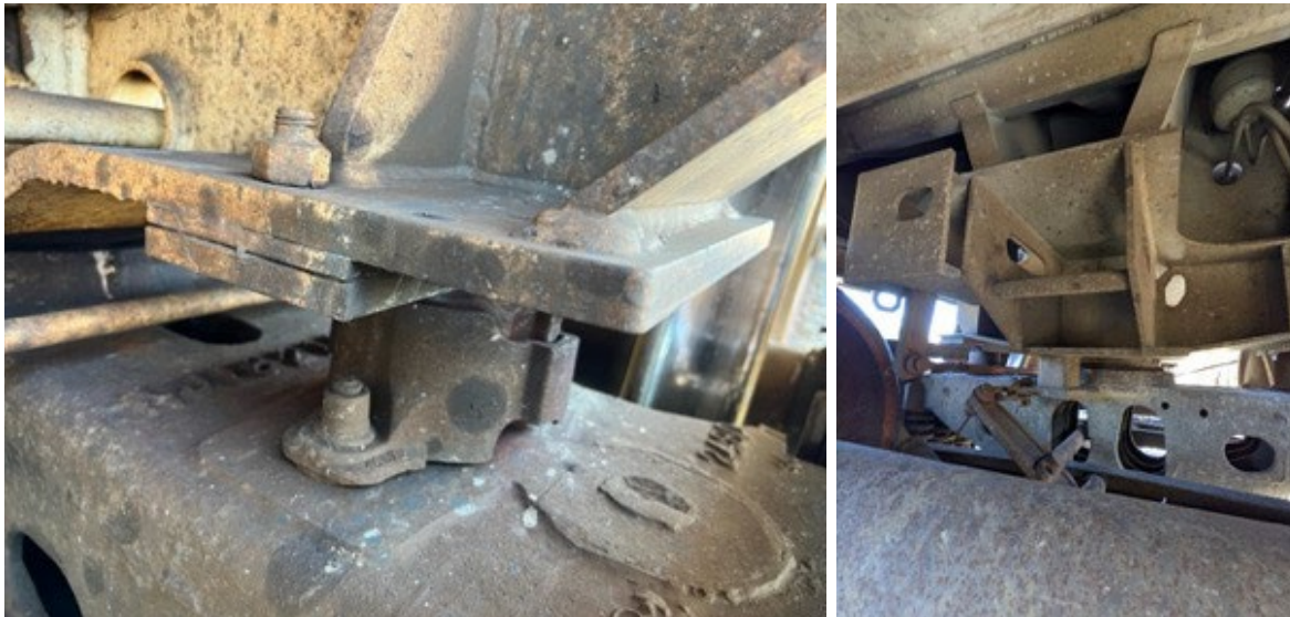
Figure 6. The Point of Contact between the Train Car and the Truck
