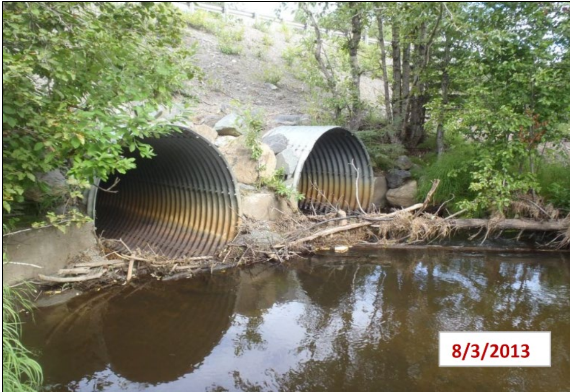
Figure 4. Observed debris at inlets during 2013 inspection.
