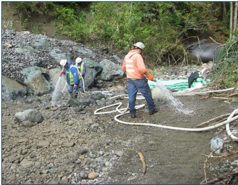
Figure 7. Construction of streambed and watering in fine sediments (SR 202 Tokul Creek, Washington). Photo by Casey Kramer.
