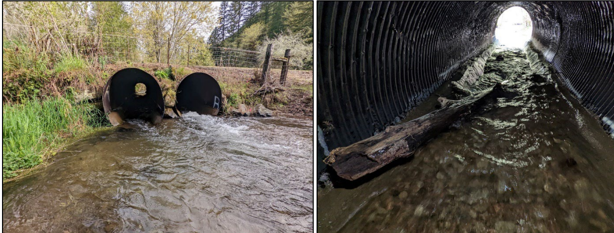
Figure 5. Looking upstream at culvert outlet (left) and looking downstream in right culvert (right).
