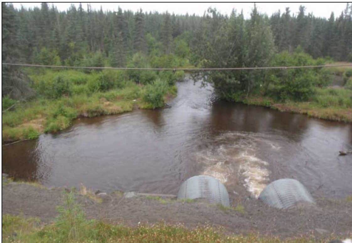
Figure 3. Scour hole during 2017 inspection.
