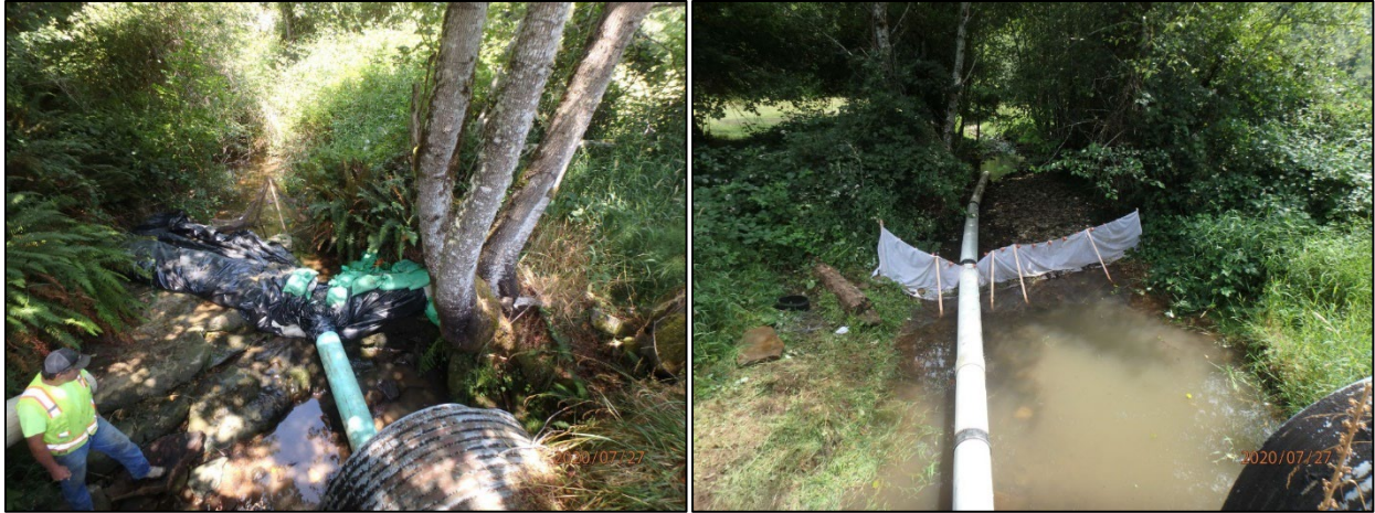
Figure 3. Upstream berm and diversion pipe (left) and downstream diversion pipe and block net (right).
