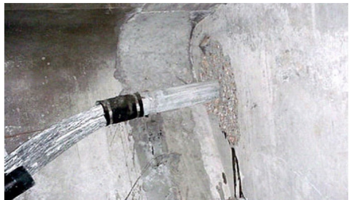
Figure 3. Photo. Failed tendon in the Mid-Bay Bridge (main cause: chloride). (4)
