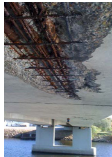
B. Exterior condition.
