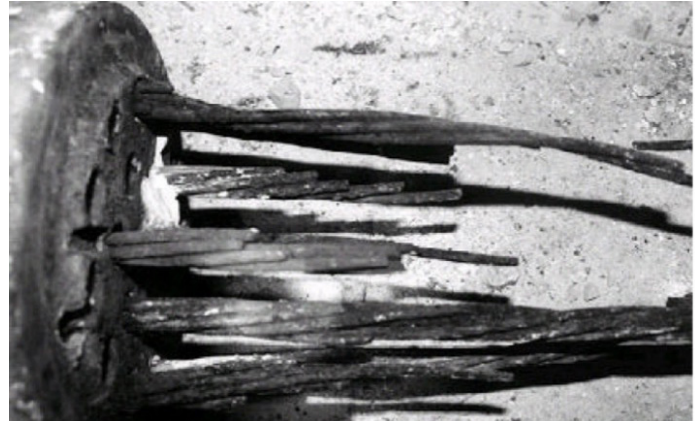
Figure 2. Photo. Failed tendon in the Niles Channel Bridge (main cause: chloride). (4,5)
