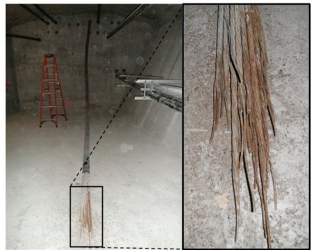
Figure 7. Photos. Ringling Causeway Bridge's first failed tendon (main cause: defective grout). (21)
