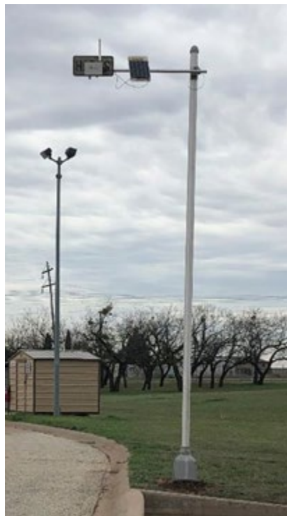
Figure 6.1: Sadeem WSS in the Abilene District maintenance yard
