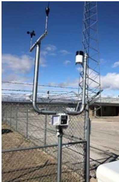
Figure 6.2: RX3000 weather station installed at a TxDOT facility in the Abilene area
