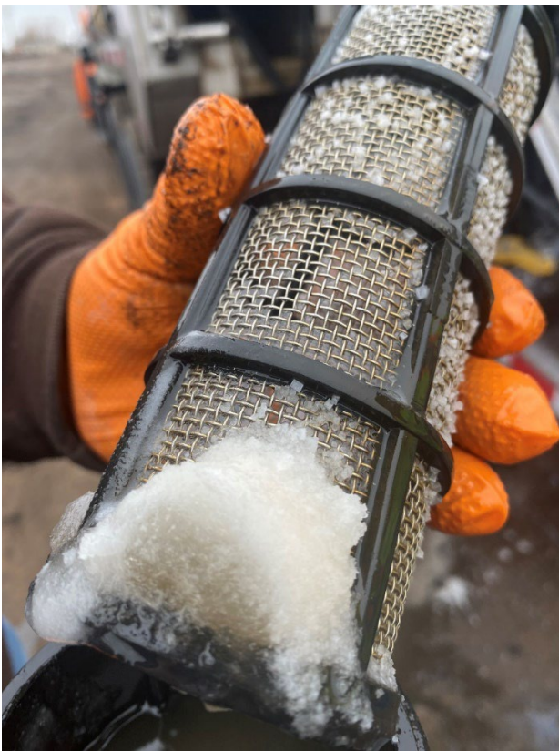
Figure 6. Screen filter clogged with salt crystals.
