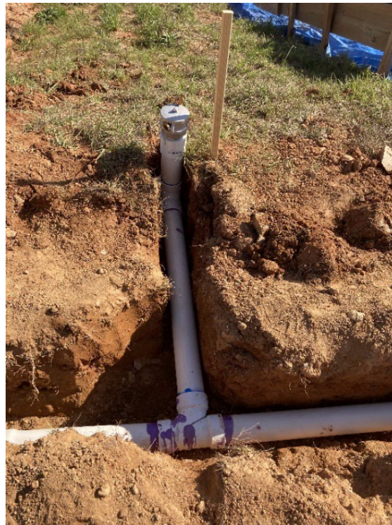
Figure 3-15: Supply Pipe Outlet
