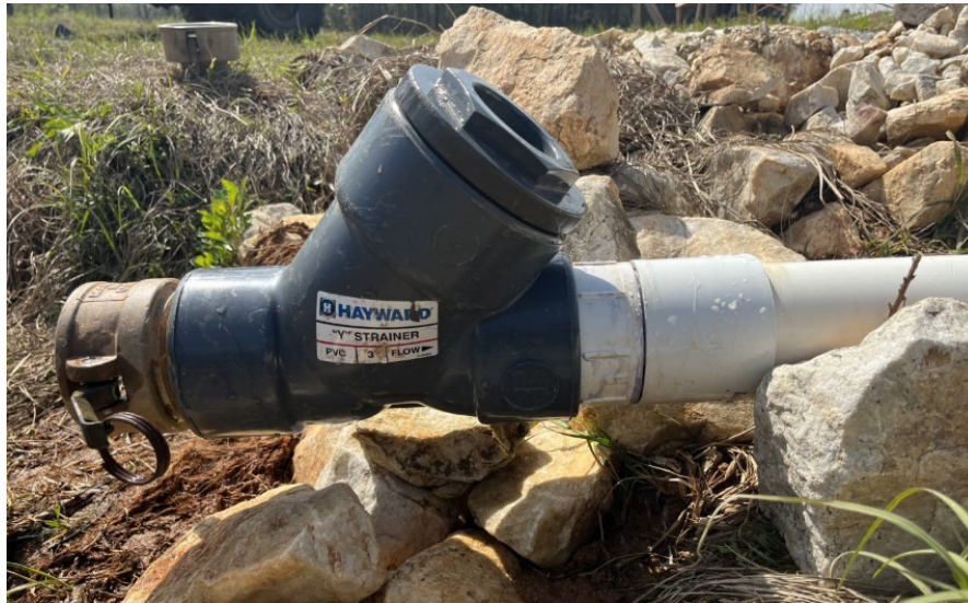
Figure 3-18: Supply Pipe Intake Debris Filter
