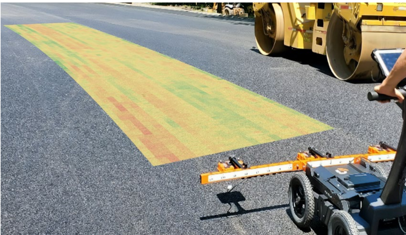
Density profiling using GPR shows advantages in obtaining continuous density measurements for large paving areas at near-real time.
