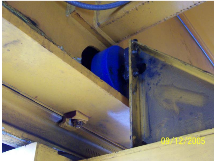
Figure 7. Photo. Return wheel running on flange.
