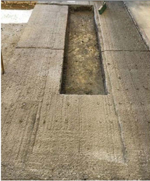
Figure 5.3 Flexible section after milling 2 in. from the surface and excavating the DWPT unit geometrical space.
