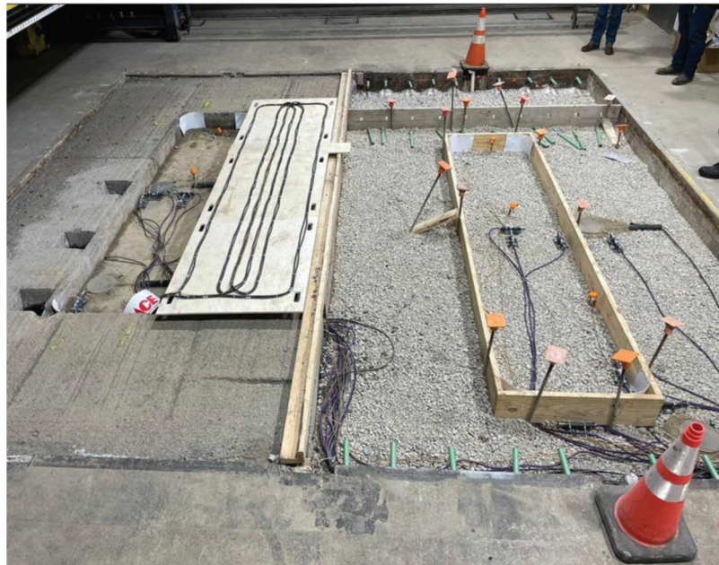
Figure 4.7 Top view of both test sections of the DWPT unit prior to material placement.
