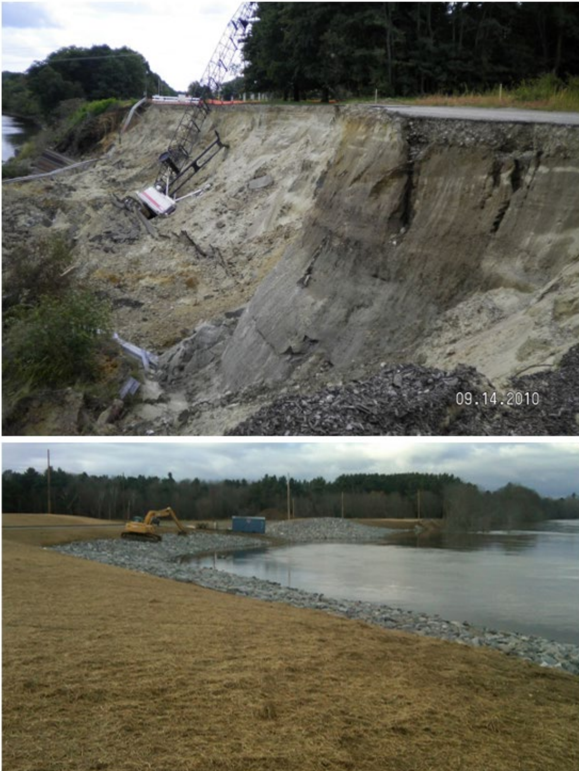
Figure 16: Project Photographs for Route 136 Slope Failure
