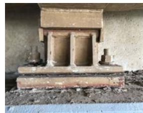
Bearing before washing
