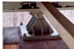
Bearing after washing
