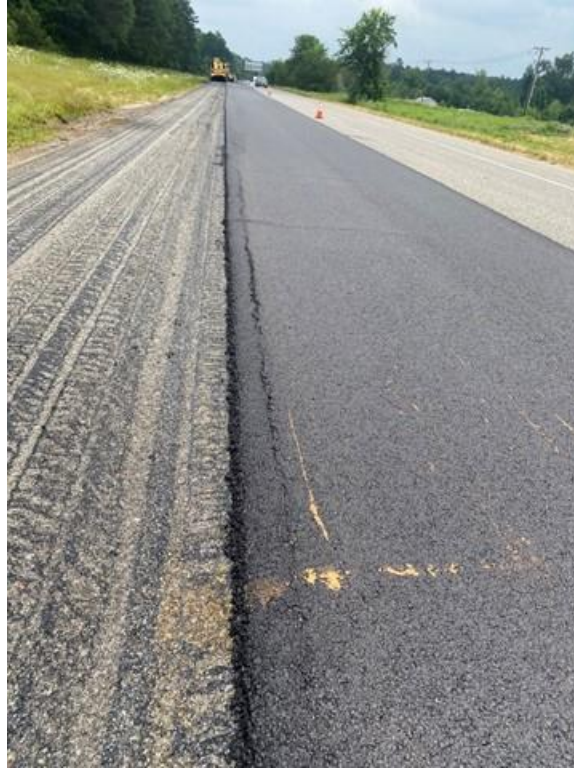
Figure 104. Bulges and cracking appearing after additional rolling in an isolated section.
