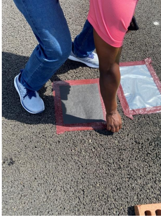
Figure 93. Roofing paper (left) and plastic sheeting (right) taped to the PFC surface.
