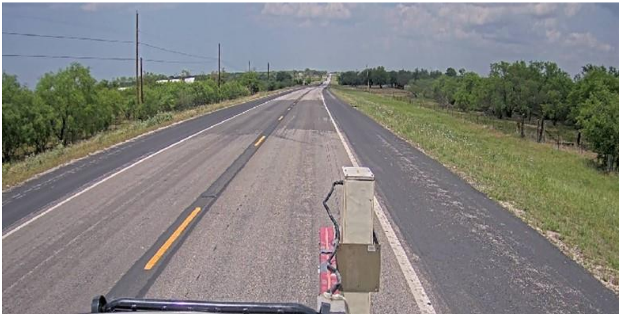
Figure 113. Several level-up cold-mix patches located throughout the project.
