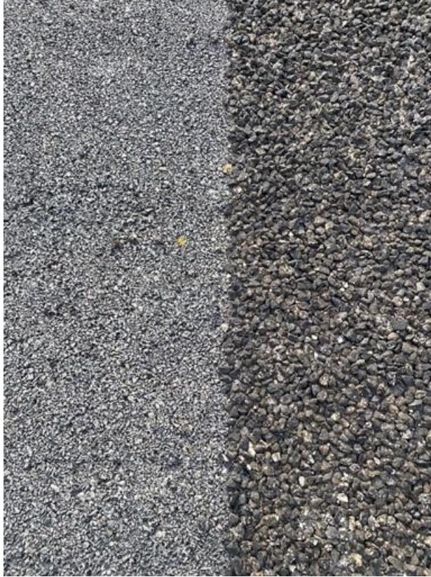
Figure 119. Close-up of seal coat next to PFC surface.
