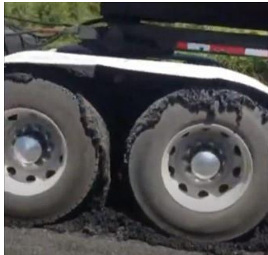
Figure 14. PFC pavement surfaced with AR seal coat tracking on vehicle tires immediately after construction.
