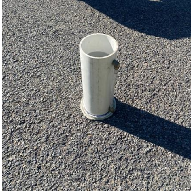
Figure 56. No water flowing in old PFC.
