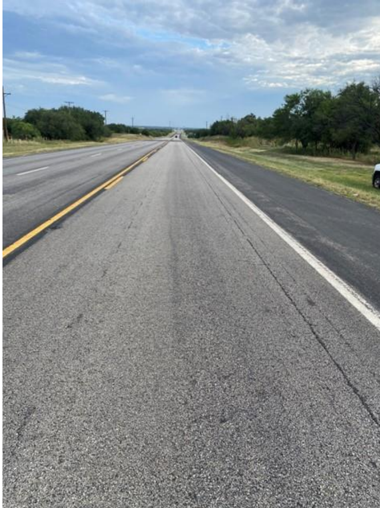
Figure 111. PFC in March of 2023 prior to seal coat showing typical distresses and evidence of the Onyx still visible on shoulder.
