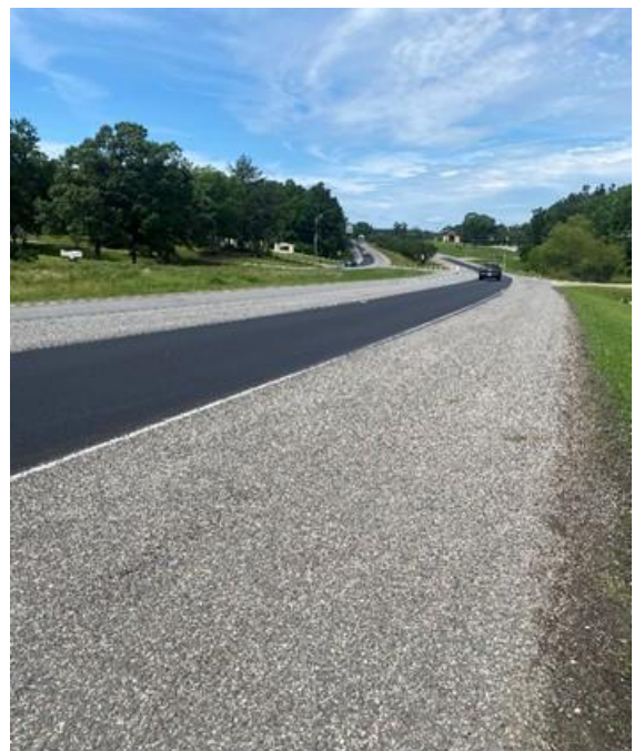
Figure 9. PFC repaired with inlaid, dense-graded hot-mix asphalt since PFC on shoulder was clogged.
