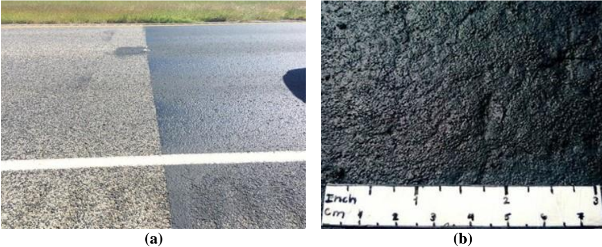
Figure 9. IH 35 in the San Antonio District: (a) beginning of Onyx product application, and (b) surface of the pavement after Onyx application (Scullion et al. 2020).
