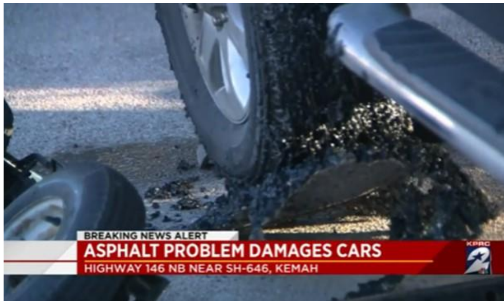
Figure 49. Seal coat causing damage to cars and tires (from TV news report).
