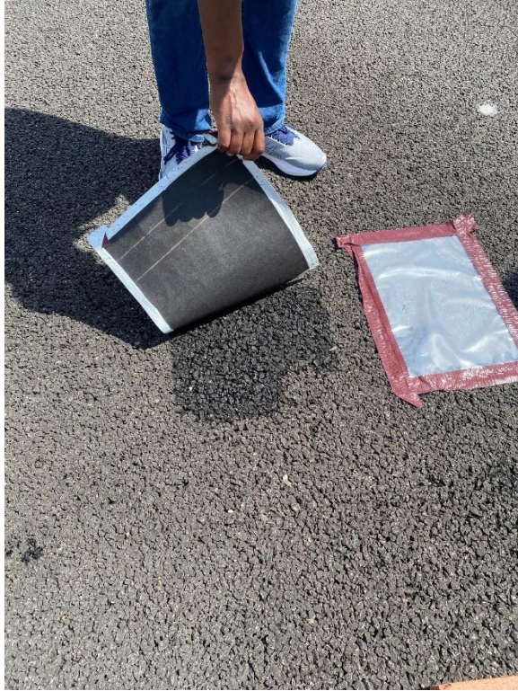
Figure 95. Moisture condensation on the underside of the roofing paper.
