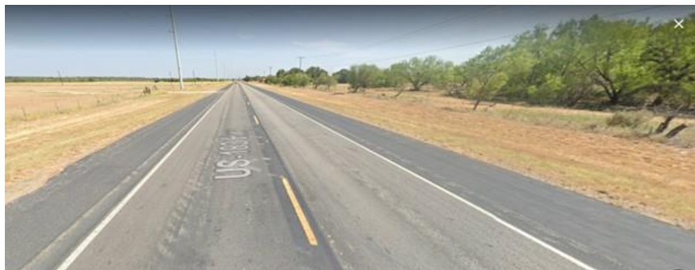
Figure 70. Condition of US 183 PFC from July 2022, Google Maps.
