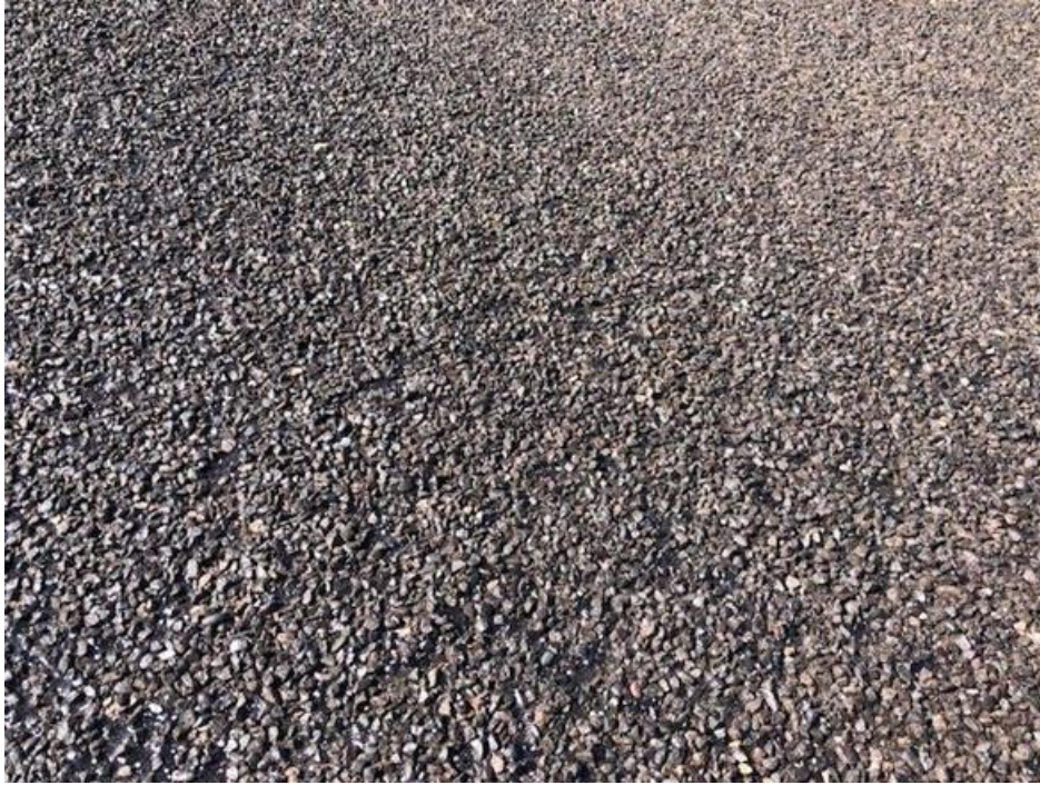
Figure 41. Seal coat at time of construction on US 90 in El Paso District.
