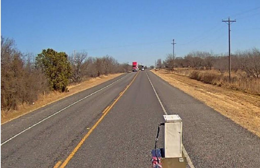
Figure 35. Current condition of seal coat on SH 36 in Brownwood District (February 2022).
