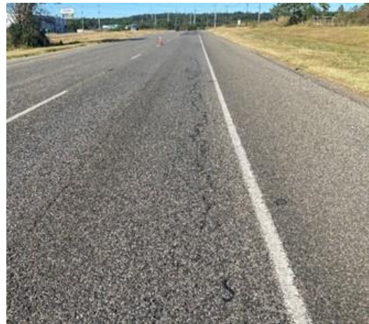
Figure 2. Cracking distress in aged PFC.
